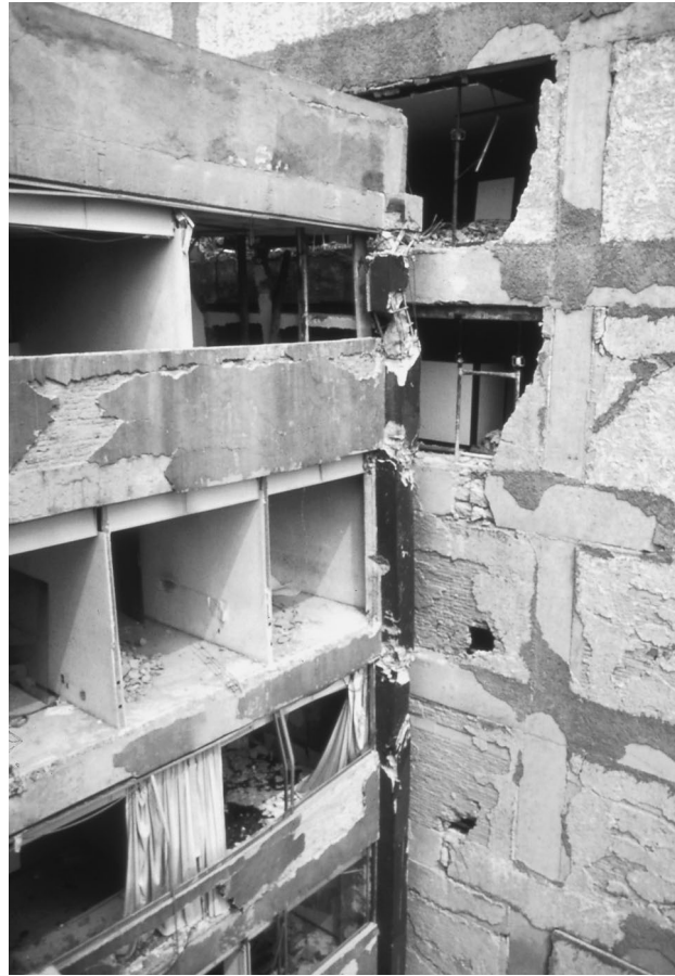
FIGURE 20.7 Damage caused by hammering for buildings with inadequate separation in the 1985 Mexico City earthquake. (Photograph courtesy of Jack Moehle)
