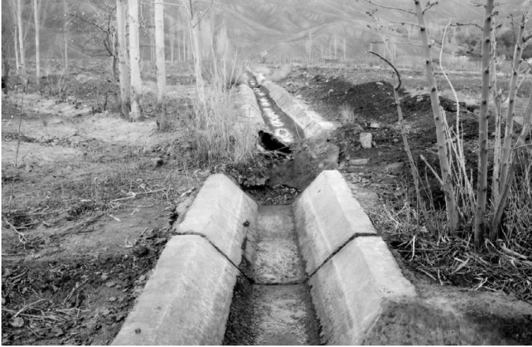
PLATE 14.6 The 14 March 1998 M_w 6.6 Fandoqā earthquake right-lateral strike-slip surface rupture of a concrete canal east of Fandoqā. The canal was earlier displaced by the 28 July 1981 M_w 7.0 Sirch earthquake and was repaired 17 years earlier, when it ruptured again by the 1998 event. See also Figure 14.1 . Courtesy of the photograph pool of Berberian et al. (2001).
