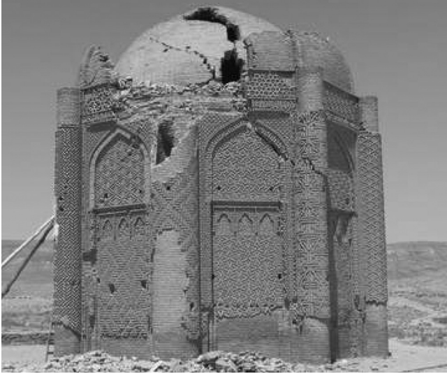
PLATE 14.14 The eleventh-century Kharaqān tomb-tower monument, damaged (VIII) during the 22 June 2002 M_w 6.4 Changureh earthquake, indicating a minimum regional seismic quiescence of about 935 years for a medium-magnitude earthquake. See Figure 14.5 and Plate 14.13. Courtesy of GSI Website; http://gsi.ir/General/Lang_en/Page51 .
