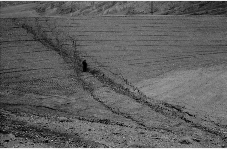
PLATE 14.4 The 14 March 1998 M_w 6.6 Fandoqā earthquake right-lateral strike-slip surface rupture of the earth dam ( 30^{\circ}00'05.13''N – 57^{\circ}40'51.17''E , +2071 m) located about 1.7 km to the south of Fandoqā playa (for location see Plate 14.1 , and Figure 14.1 ). View to the northeast. Courtesy of the photograph pool of Berberian et al. (2001).
