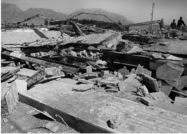
PLATE 13.32 Complete collapse of the reinforced concrete structures at Ardekul during the 10 May 1997 M_w 7.2 Zirkuh earthquake. See Figures 13.17 and 13.18 for the location, fault, and meizoseismal area of the earthquake. The collapsed buildings were constructed after the 14 November 1979 M_w 6.6 Korizān earthquake. Photographed in May 1997. View to the north.
