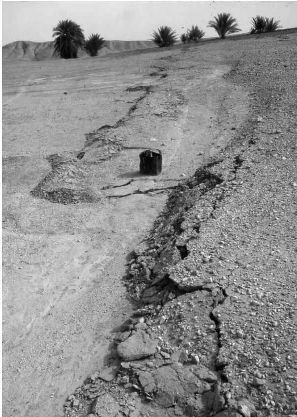
PLATE 13.12 Coseismic thrust faulting associated with the 16 September 1978 M_w 7.3 Tabas-e Golshan earthquake, southeast of Tabas-e Golshan. Looking north. See also Figure 13.8. Photographed in September 1978 (Berberian, 1979a).
