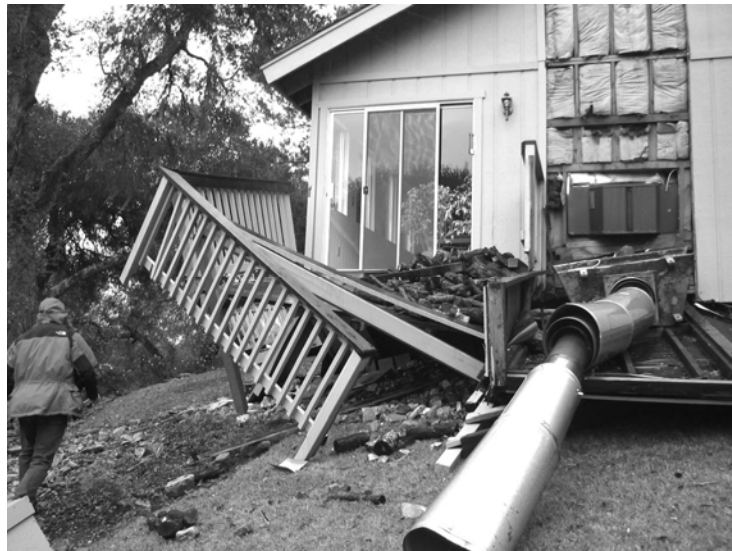
Figure 7-8 Collapsed factory-built chimney, light-frame enclosure, and deck after the San Simeon earthquake. Photo courtesy of Josh Marrow, Simpson Gumpertz and Heger Inc.
