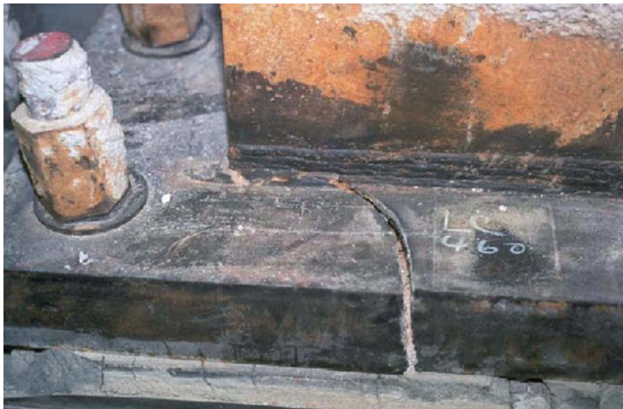
Figure 11-1 Fractured 4-inch-thick steel base plate, university building, Northridge, 1994. (photo courtesy of the Earthquake Engineering Research Institute)
