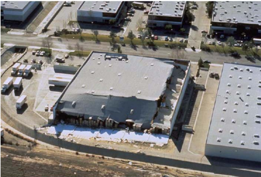
Figure 8-1 Roof and wall collapse of tilt-up building during the 1994 Northridge earthquake. (Photo courtesy of the Earthquake Engineering Research Institute)
