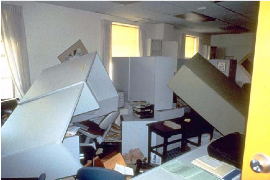
Figure 6-1 Typical earthquake damage to contents and nonstructural components in a modern office building. (photo courtesy of the Earthquake Engineering Research Institute)
