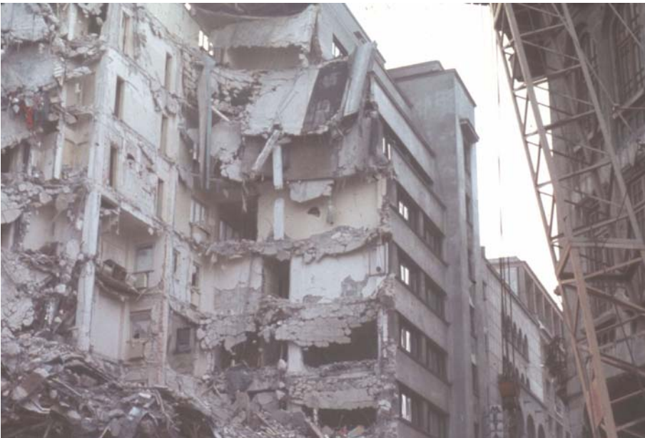
Figure 3-4 Preseismic-code ten-story reinforced-concrete-frame building in Bucharest, Romania, that partially collapsed during the 1977 magnitude-7.2 earthquake approximately 65 miles north of Bucharest. (photo courtesy of C. Rojahn)
