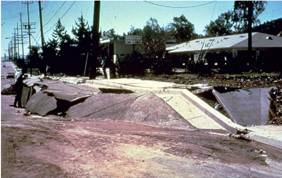
Figure 3-8 Example of surface fault rupture; 1971 San Fernando, California, earthquake (a thrust fault earthquake). (Photo courtesy of the Earthquake Engineering Research Institute.)
