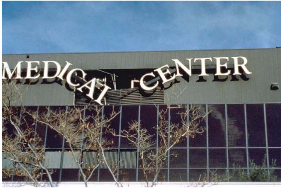
Figure 9-1 Exterior view of Holy Cross Medical Center, which was evacuated after the 1994 Northridge earthquake due to damage to the HVAC system. (photo courtesy of the Earthquake Engineering Research Institute)
