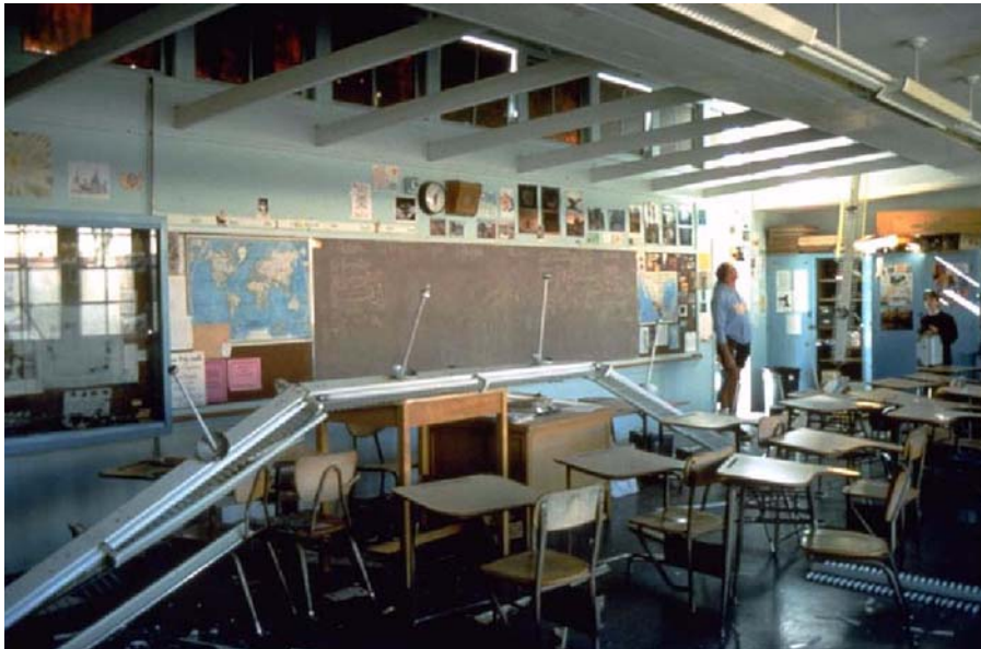
Figure 10-1 Nonstructural damage at Northridge Junior High where lights fell onto desks during the 1994 Northridge earthquake. (photo courtesy of the Earthquake Engineering Research Institute)
