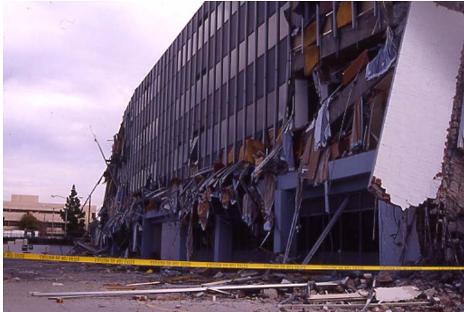
Figure 6-2 Exterior view of medical office building severely damaged by the 1994 Northridge earthquake. (C. Arnold photo)
