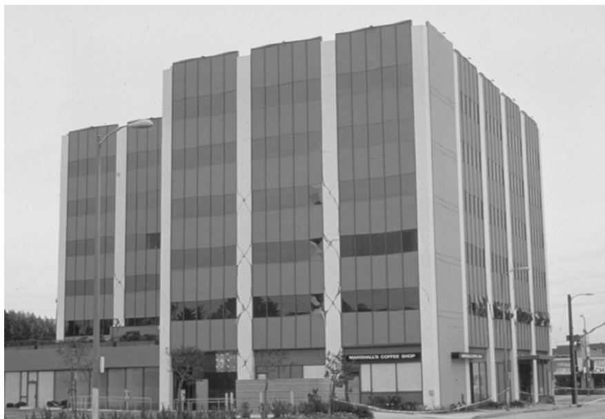
Figure 3-1 Six-story concrete-moment-frame medical building that was severely damaged by the magnitude-6.8 Northridge, California, earthquake of January 17, 1994. The building was subsequently demolished without removing contents. (photo courtesy of the Earthquake Engineering Research Center, University of California at Berkeley)
