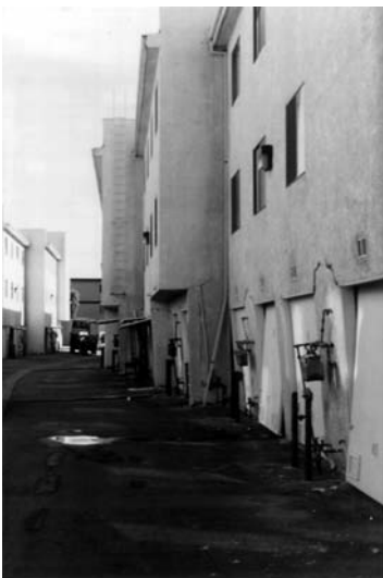
Relatively new apartment complex damaged in the 1994 Northridge Earthquake
