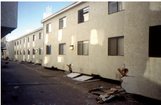
Figure 8-5: A tuck-under similar to Figure 8-4, but much more modern and designed at a time when the weakness of the parking level was more understood. In this case, the detailing of the small wood shear walls at that level was poor. This practice created another set of deficient “existing” buildings.
