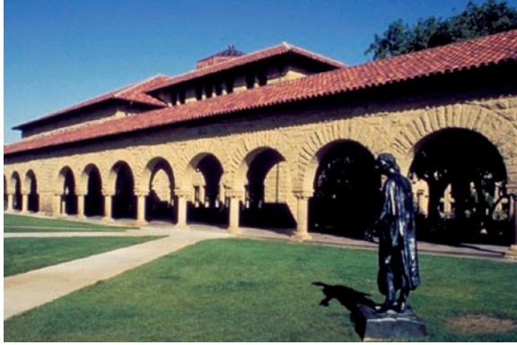
Figure 8-24: Original Quad arcades, Stanford University. The Quad, approximately 850 feet by 950 feet in plan, is surrounded by a covered arcade. Modern seismic retrofits have taken place over a 40-year period, with evolving techniques. Final sections were completed by removal of the interior wythe of sandstone, installation of reinforced concrete core, and reinstallation of the interior blocks, which were reduced in thickness. Due to environmental decay of many of the sandstone columns, additional seismic resistance was obtained in many locations by installation of precast concrete replicas that formed a part of a continuous vertical reinforced concrete member.
