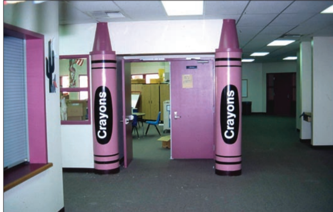
Figure 9-2: Limited nonstructural damage at Landers Elementary.
