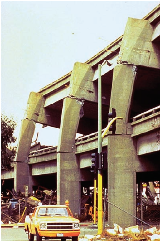
Figure 6-6: San Francisco, 1989, elevated highway support bents, an example of failure of engineered structures.
