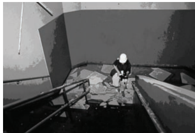
Figure 9-6: Difficulty in exiting due to debris strewn across exit stairs can be an indirect threat to life, as can be seen in this photo following the Loma Prieta earthquake in 1989.
