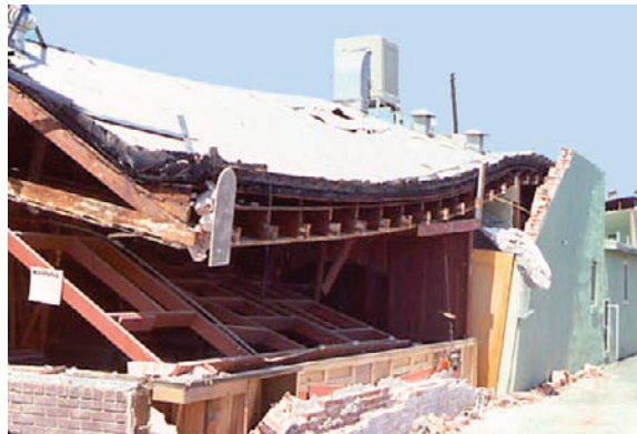
Figure 8-1: Example of buildings with no code design. Damage shows classic URM deficiencies.
