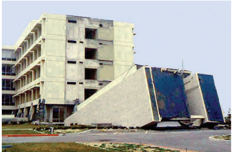
Figure 8-2: Olive View Hospital. A brand new facility that was damaged beyond repair in the 1971 San Fernando earthquake due to a shaking intensity that exceeded what was expected at the site and a design that, although technically complying with code at the time, contained several structural characteristics now considered major deficiencies. The lateral system contained nonductile concrete frames, discontinuous shear walls, and a significant weak story.
