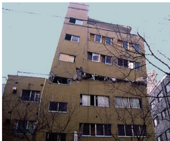
Figure 5-30 Damaged building, Kobe earthquake, Japan, 1995.
