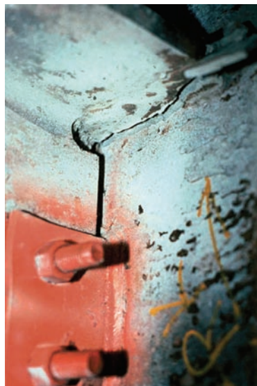
Figure 6-7: Northridge, 1994 Failure of a welded steel connection.
