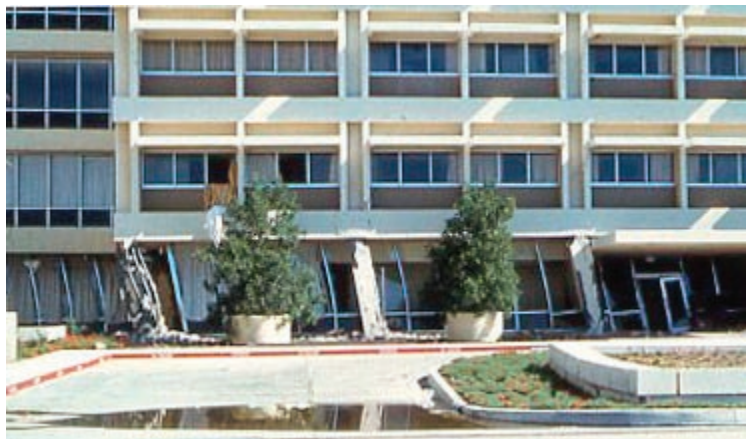
Figure 5-15: Olive View hospital, San Fernando earthquake, 1971, showing the extreme deformation of the columns above the plaza level.
