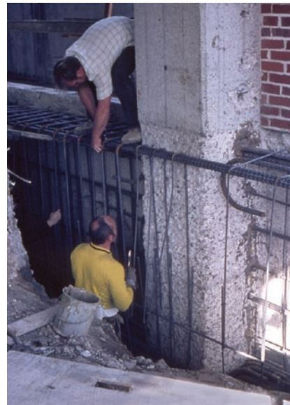
Figure 8-11: Retrofit activities inside buildings are most often not surgical or delicate. Here work on a new foundation for a shear wall is prepared for casting.
