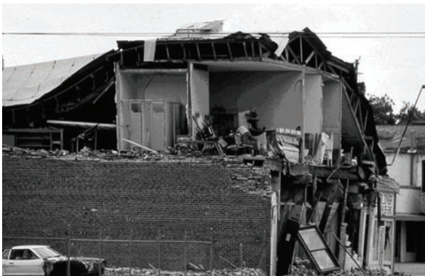
Figure 9-4: Nonstructural partition walls prevented the total collapse of this unreinforced masonry structure in the 1983 Coalinga earthquake.
