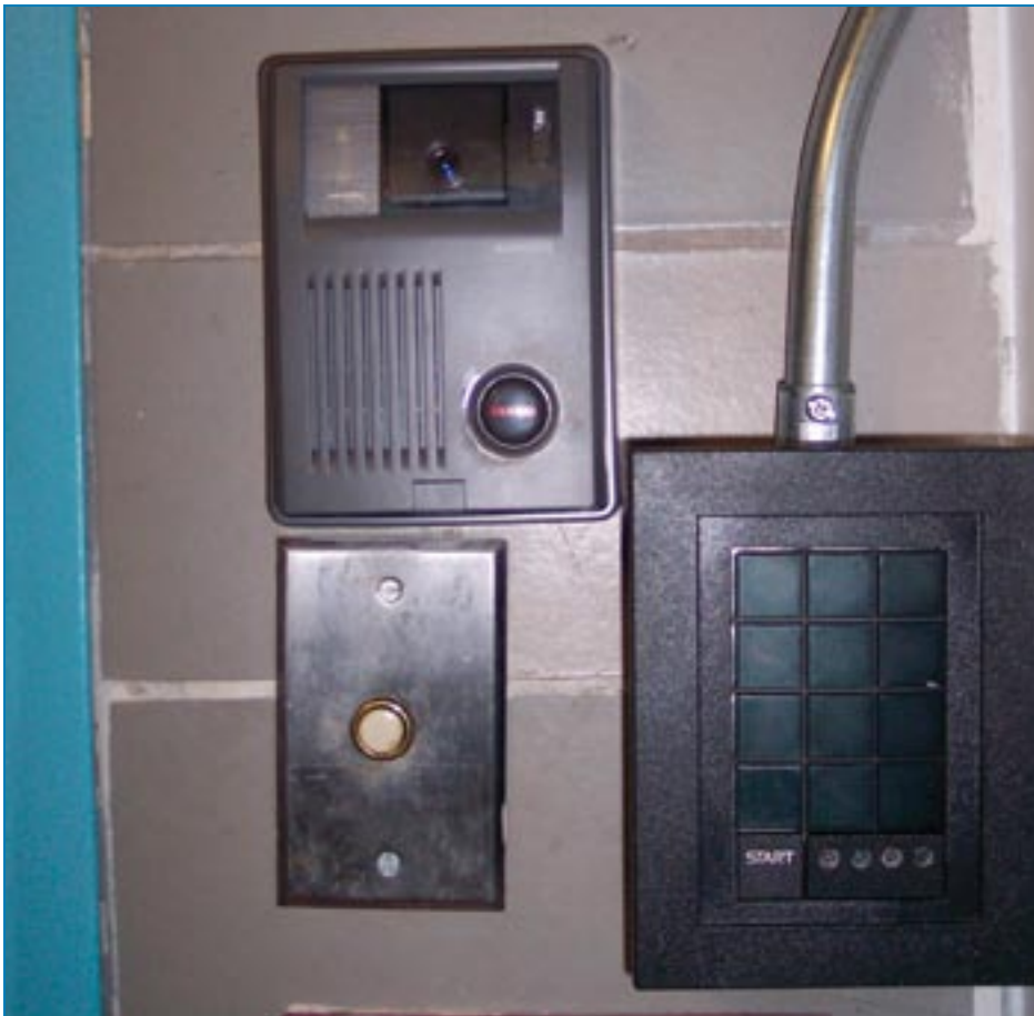
Figure 5-7: Electronic entry control device into restricted area. SOURCE: BOB CIZMADIA
