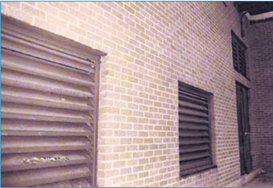
Figure 4-3: Typical air intakes.
