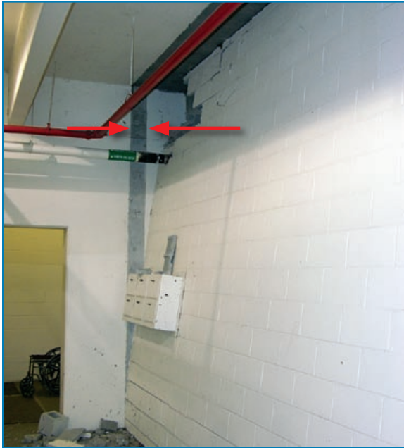
Figure 3-44: The red arrows show the original location of a CMU wall that nearly collapsed following a rolling door failure. Hurricane Charley (Florida, 2004)
