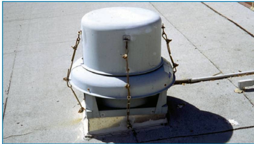
Figure 3-71: Cables were attached to prevent the cowling from blowing off. Typhoon Paka (Guam, 1997)
