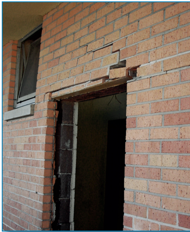
Figure 2-28: Brick facing separated from the masonry wall at Port Sulpher High School, LA.
