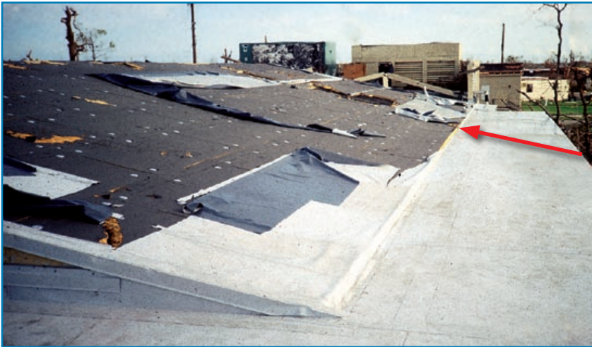
Figure 3-89: Mechanically attached single-ply membrane progressively tore after being cut by wind-borne debris. Hurricane Andrew (Florida, 1992)
