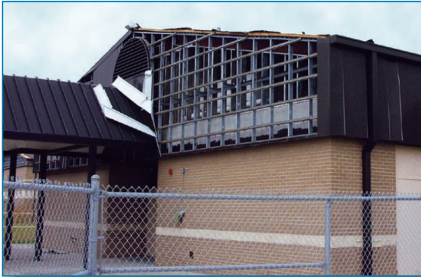
Figure 3-58: The loss of metal wall panels allowed a substantial amount of wind-driven rain to penetrate this building. Hurricane Ivan (Florida, 2004)
