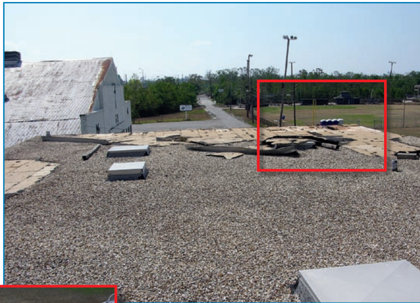
Figure 3-115: The built-up roof on this school was blown off after a few of the rotted wood planks detached from the joists. Hurricane Katrina (Mississippi, 2005)
