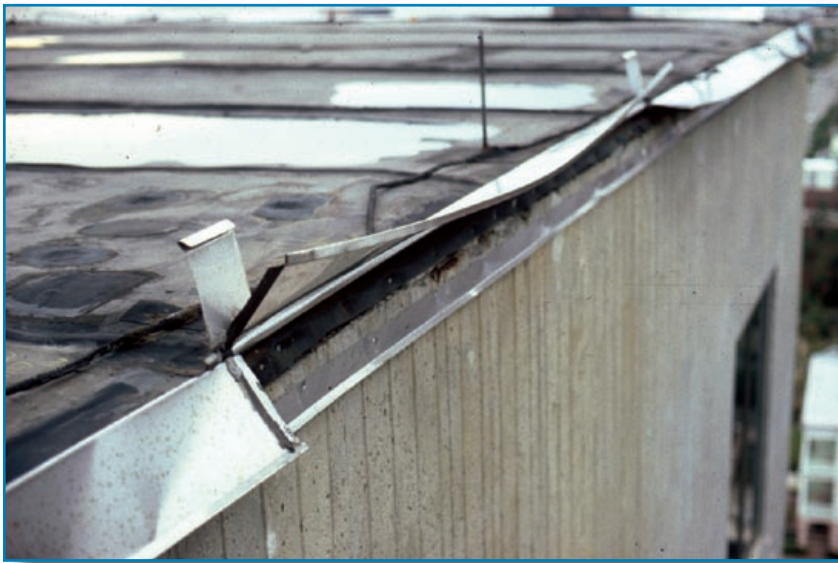
Figure 3-62: The metal edge flashing disengaged from the continuous cleat and the vertical flange lifted. Hurricane Hugo (South Carolina, 1989)
