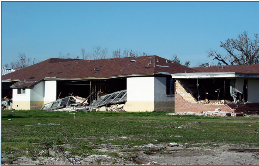
Figure 4-29: Damaged non-load-bearing walls at Charles B. Murphy Elementary School
