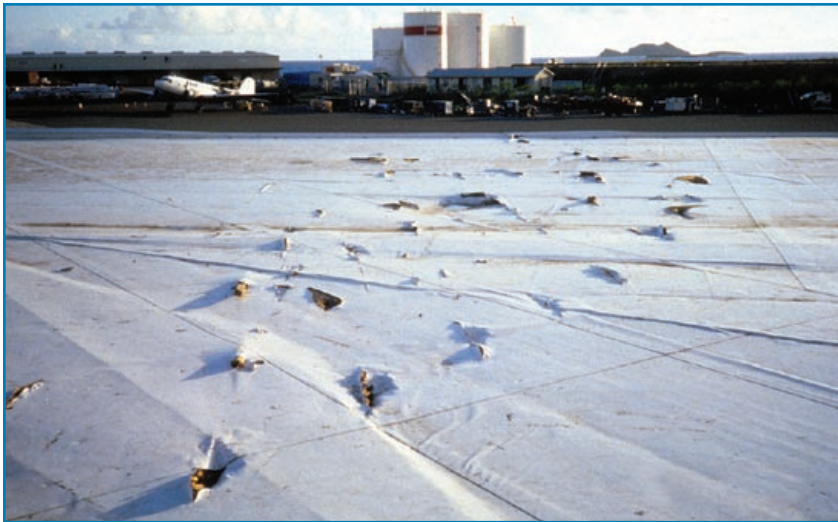
Figure 3-90: Fully adhered single-ply roof membrane struck by a large number of missiles. Hurricane Marilyn (U.S. Virgin Islands, 1995)
