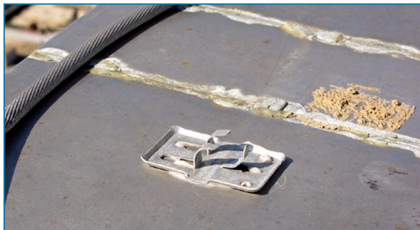
Figure 3-96: The conductor deformed the prongs under wind pressure, and pulled away from the connector. Hurricane Katrina (Mississippi, 2005)
