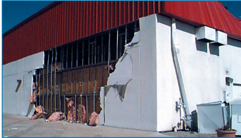
Figure 3-54: EIFS blow-off at building corner. In places, metal fascia was also blown in. Tornado (Oklahoma, 1999)
