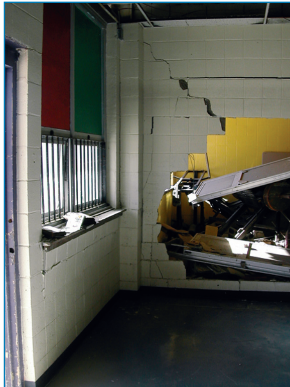
Figure 2-14: Interior unreinforced masonry walls of the Port Sulphur High School in Louisiana were damaged by hydrostatic loads associated with Hurricane Katrina's storm surge (2005).
