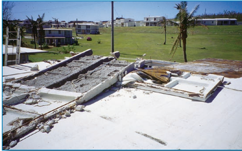
Figure 3-26: Portions of this waffled precast concrete roof deck were blown off. Typhoon Paka (Guam, 1997)
