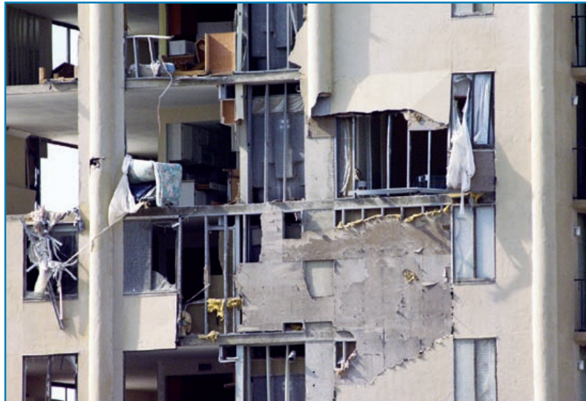
Figure 3-57: The stucco wall failure was caused by inadequate attachment between the stud tracks and the building's structure. Hurricane Ivan (Florida, 2004)
