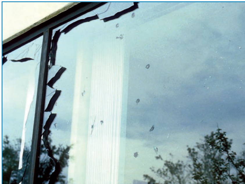
Figure 3-13: The outer window panes were broken by aggregate from a built-up roof. Hurricane Hugo (South Carolina, 1989)
