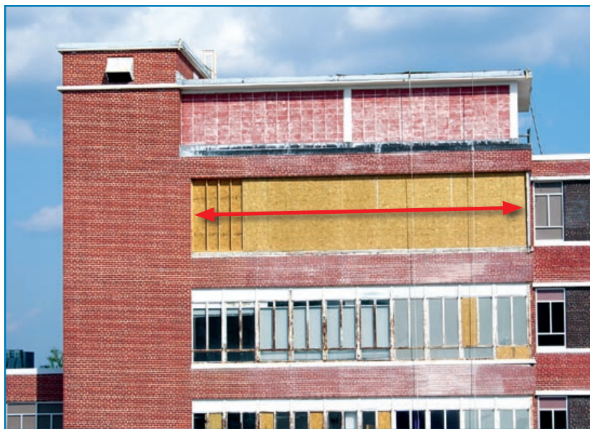
Figure 3-110: Wind pressure caused the window frames on the upper floor to fail (red arrow). Hurricane Katrina (Mississippi, 2005)
