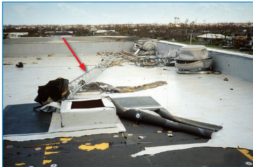
Figure 3-79: The collapse of the antenna tower caused progressive peeling of the roof membrane. Also note that the exhaust fan blew off the curb, but the high parapet kept it from blowing off the roof. Hurricane Andrew (Florida, 1992)
