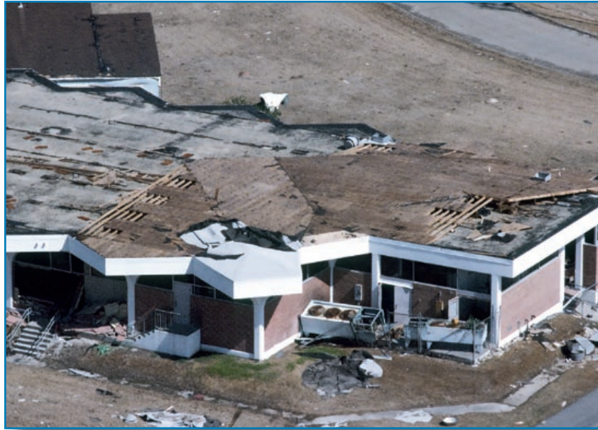
Figure 3-108: The school's wood superstructure installed as part of a steep-slope conversion blew away because of inadequate attachment. Hurricane Katrina (Louisiana, 2005)
