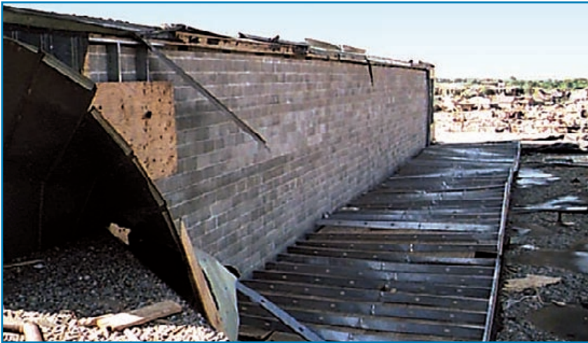
Figure 3-14: Collapsed metal stud wall—the wall was blown completely away in another part of the building. (Oklahoma, 1999)
