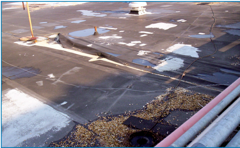
Figure 4-7: Roof membrane starting to peel off at Hancock Medical Center.
