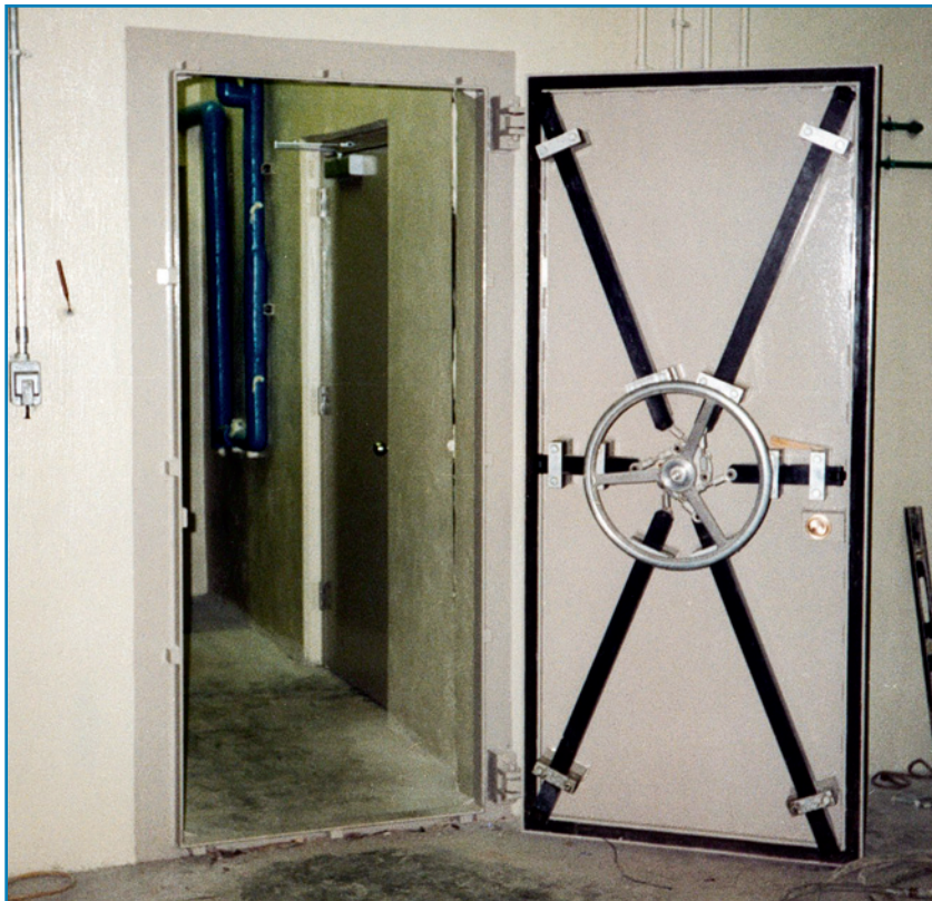
Figure 2-29: Permanent watertight doors for deep water
