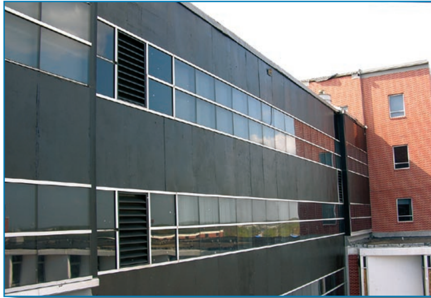
Figure 3-84: Plywood panels (black continuous bands) installed after the glass spandrel panels were broken by roof aggregate. Hurricane Katrina (Mississippi, 2005)
