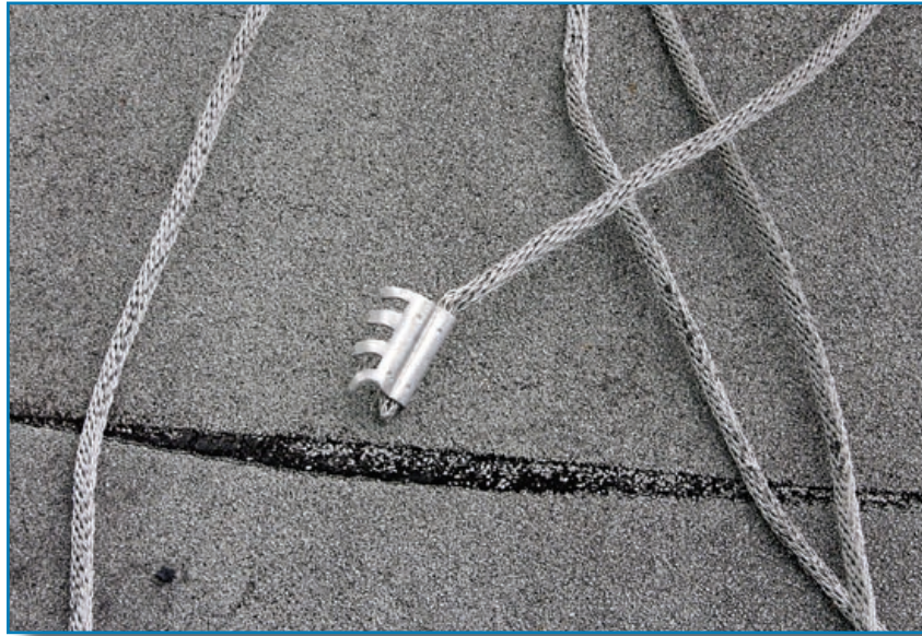
Figure 3-100: If conductors detach from the roof, they are likely to pull out from pronged splice connectors. Hurricane Charley (Florida, 2004)
