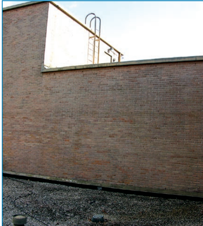
Figure 3-52: Water leaked inside along the base of the brick veneer walls. Hurricane Katrina (Louisiana, 2005)
