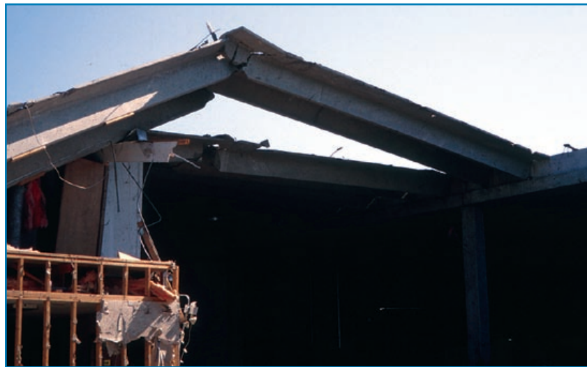
Figure 3-27: Twin-Tee roof panel lifted as a result of the combined effects of wind uplift and pre-tension. Tornado (Missouri, May 2003)
