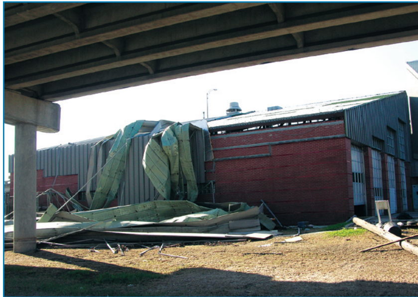
Figure 4-42: Metal roof and wall panels peeled off the Third District Fire Station in New Orleans
