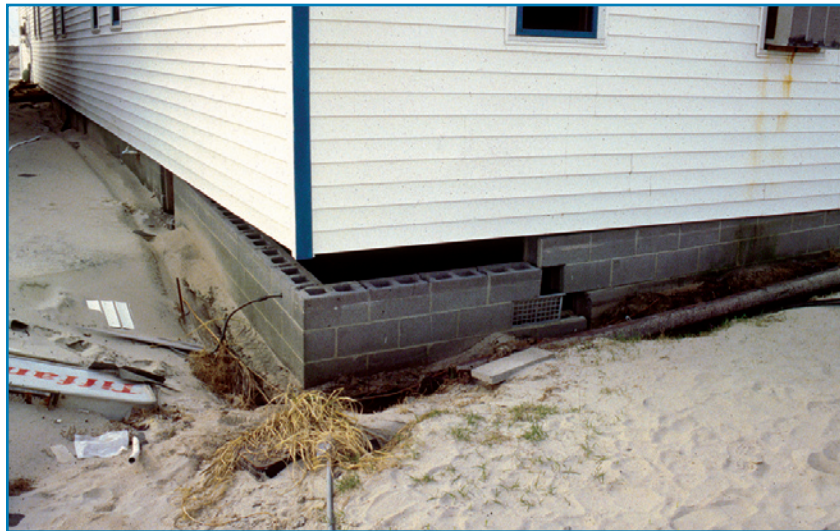
Figure 2-11: Local scour undermined this shallow foundation (also note that the building was not anchored to the foundation).
