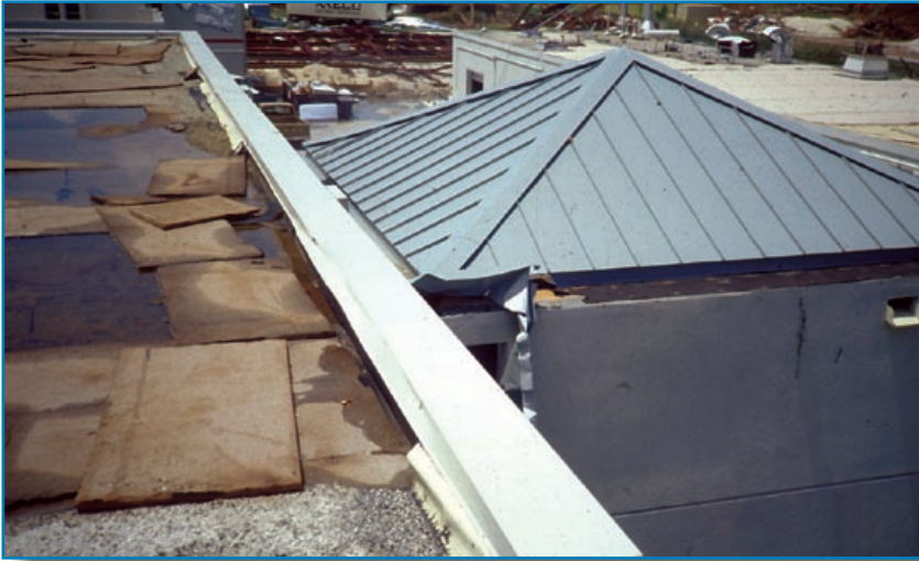
Figure 3-10: The irregularity created by the stair tower (covered with a metal roof) caused turbulence resulting in wind speed-up and roof damage. Hurricane Andrew (Florida, 1992)
