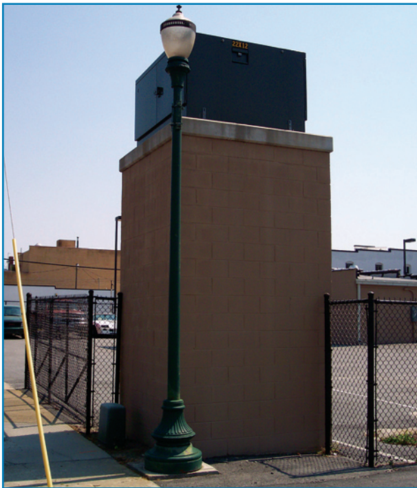
Figure 2-34: Elevated utility box
