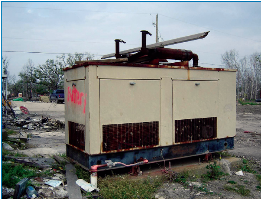
Figure 2-20: Although it was anchored and not displaced by floodwaters, this generator was out of service after being submerged.
