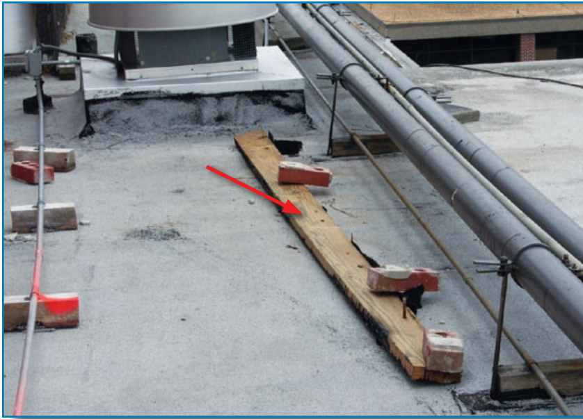
Figure 3-116: The edge nailer on top of an old brick wall at a hospital blew off because it was inadequately attached. Hurricane Ivan (Florida, 2004)
