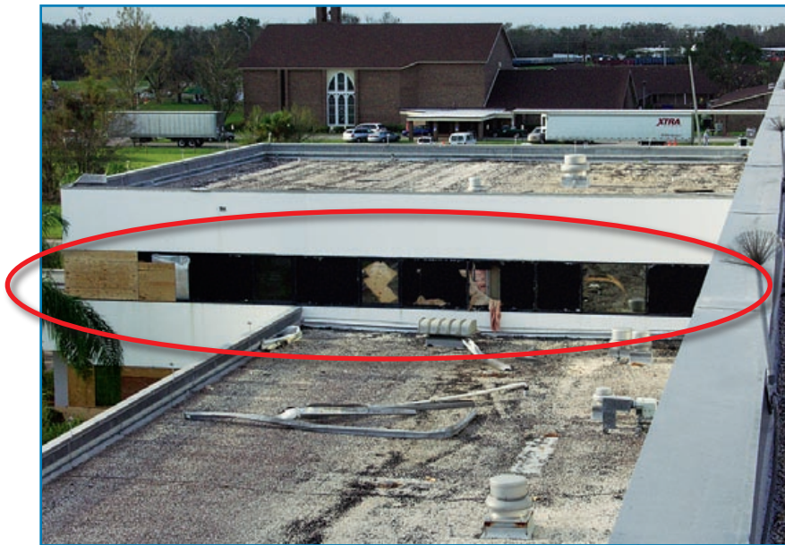
Figure 3-114: Aggregate from the hospital's built-up roofs broke several windows in the intensive care unit, which had to be evacuated during the hurricane. Hurricane Charley (Florida, 2004)
