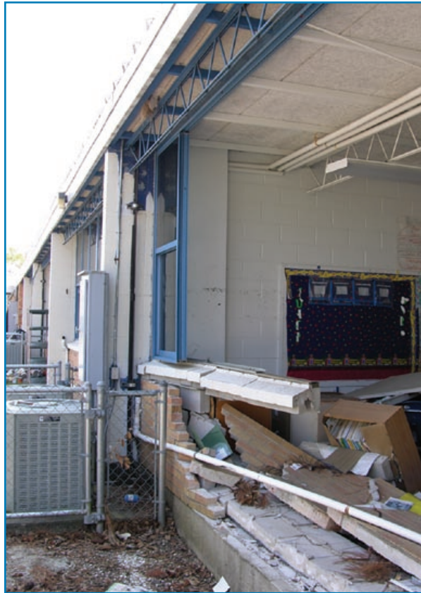
Figure 3-105: Several walls at this school collapsed. Windows were located above a non- load-bearing masonry wall. Hurricane Katrina (Mississippi, 2005)
