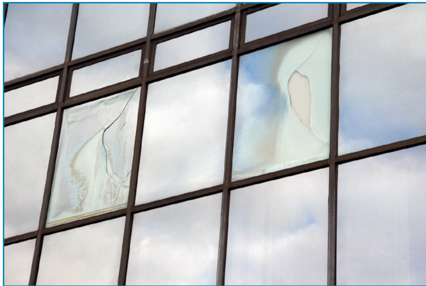
Figure 4-9: Broken windows at Touro Infirmary
