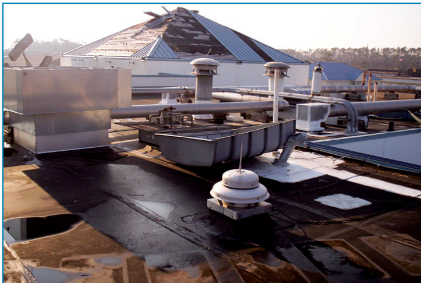
Figure 4-8: Roof damage on Hancock Medical Center
