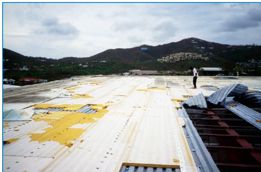
Figure 3-59: The orientation of the membrane fastener rows led to blow-off of the steel deck. Hurricane Marilyn (U.S. Virgin Islands, 1995)
