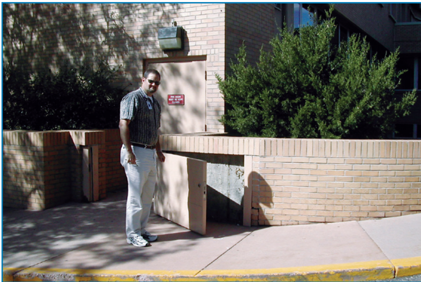
Figure 2-33: Boulder Community Hospital, Boulder, CO installed this permanently mounted floodgate in a low floodwall; the floodgate swings to the left to close off the door that leads to the mechanical equipment room.
