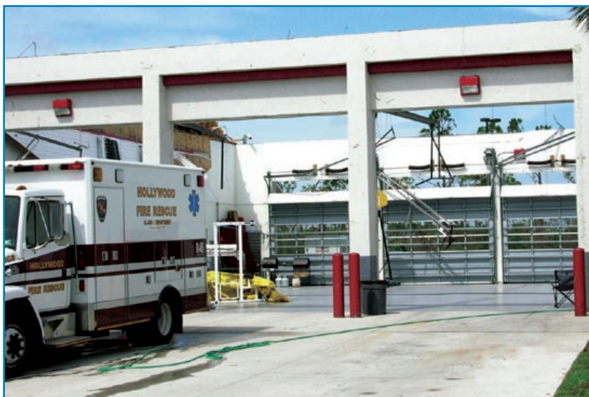
Figure 3-30: The roof structure over the apparatus bay blew off following the failure of sectional doors. Hurricane Charley (Florida, 2004)
