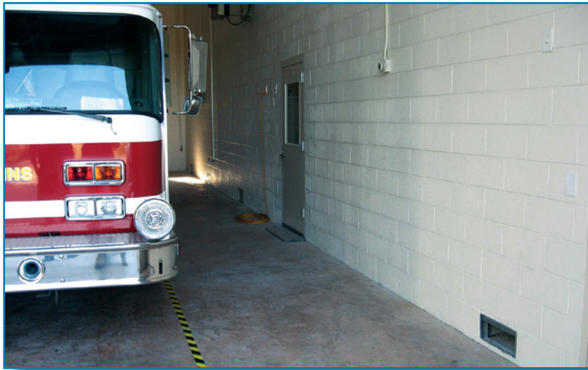
Figure 2-35: The enclosed entry and storage area to the right of the fire truck bays were retrofitted with flood openings.
