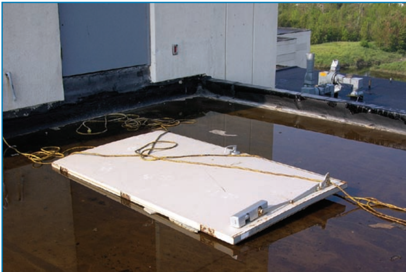
Figure 3-29: Door on a hospital penthouse blown off its hinges during Hurricane Katrina (Mississippi, 2005)
