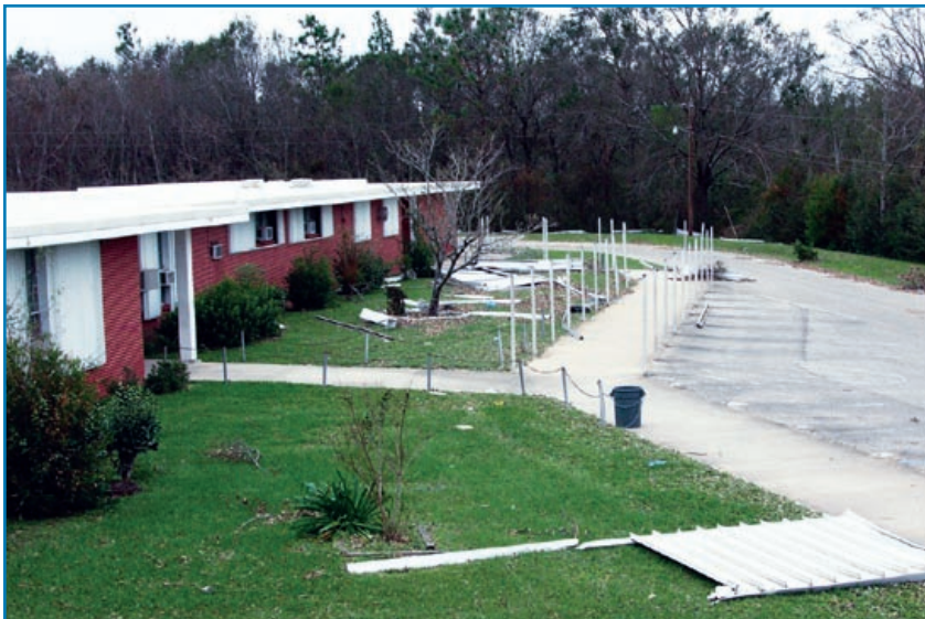
Figure 3-28: The destroyed walkway canopy in front of a school became wind-borne debris. Hurricane Ivan (Florida, 2004)
