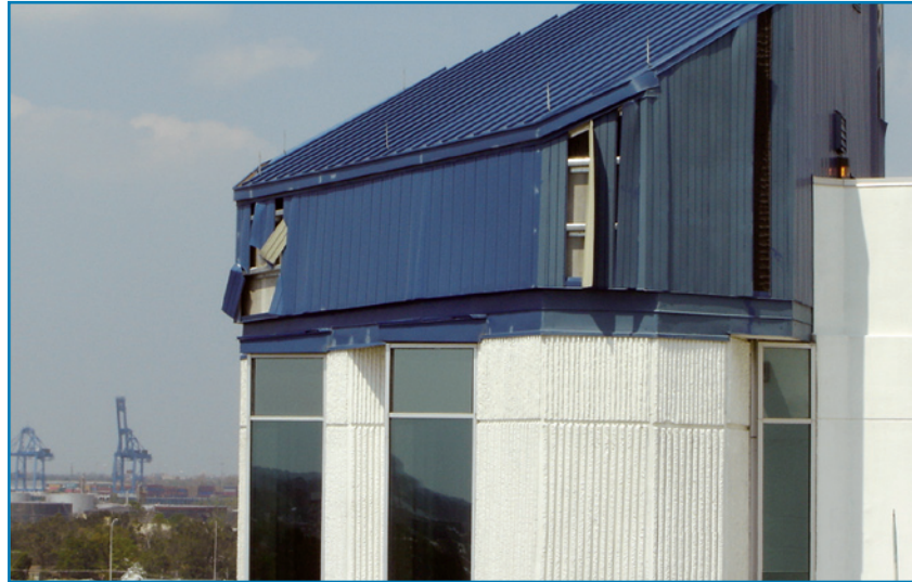
Figure 4-4: Penthouse at the West Jefferson Medical Center
