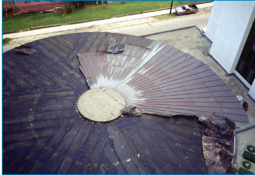
Figure 3-86: Because this roof system incorporated a secondary membrane, the ICU was not evacuated after the copper roof blew off. Hurricane Andrew (Florida, 1992)
