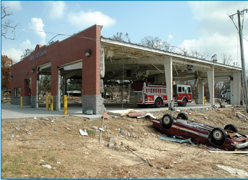
Figure 4-40: Exterior walls on the Gulfport Fire Station #7 washed away by the storm surge
