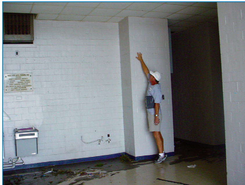
Figure 4-16: D'Iberville Middle School was flooded to the depth of 8 feet
