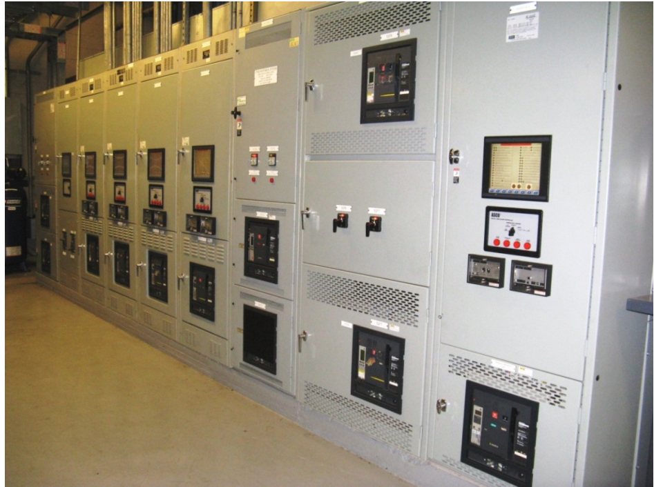
Figure 5-7 Generator synchronizing board.
