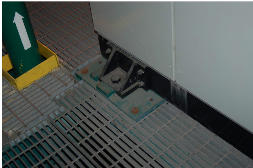
Figure 2-15 Well-anchored equipment (FEMA, 2012b).
