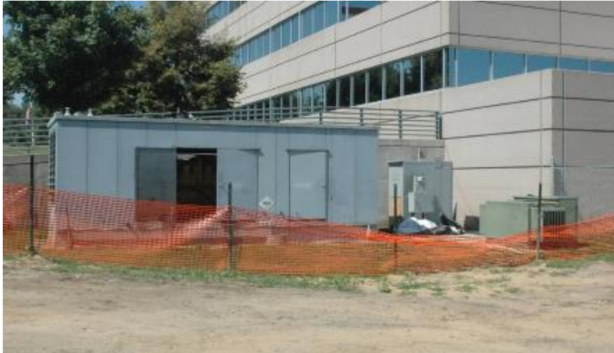
Figure 2-11 Emergency generator in an exterior enclosure in Cedar Rapid, Iowa, inundated during the 2010 Midwest floods.
