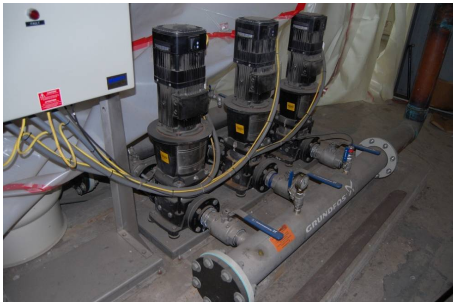
Figure 4-8 Domestic water booster pumps.
