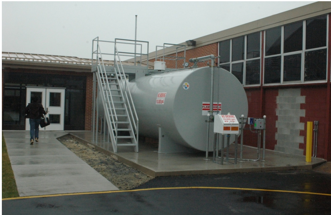
Figure 5-5 Fuel oil storage tank used for heating equipment that can supply an emergency diesel generator.
