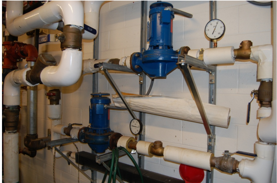
Figure 4-9 Domestic hot water circulator pumps.
