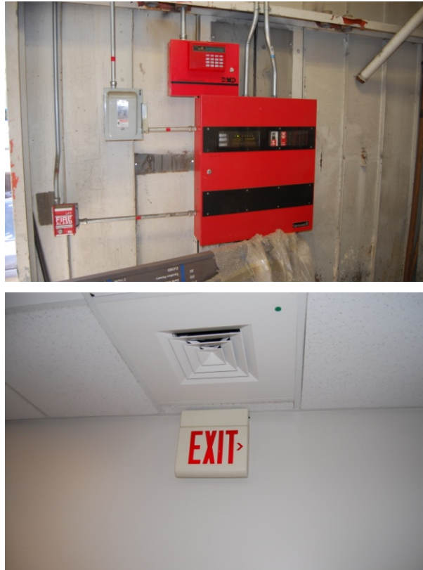
Figure 4-1 Life-safety equipment: fire alarm control panel (top) and exit signage (bottom).
