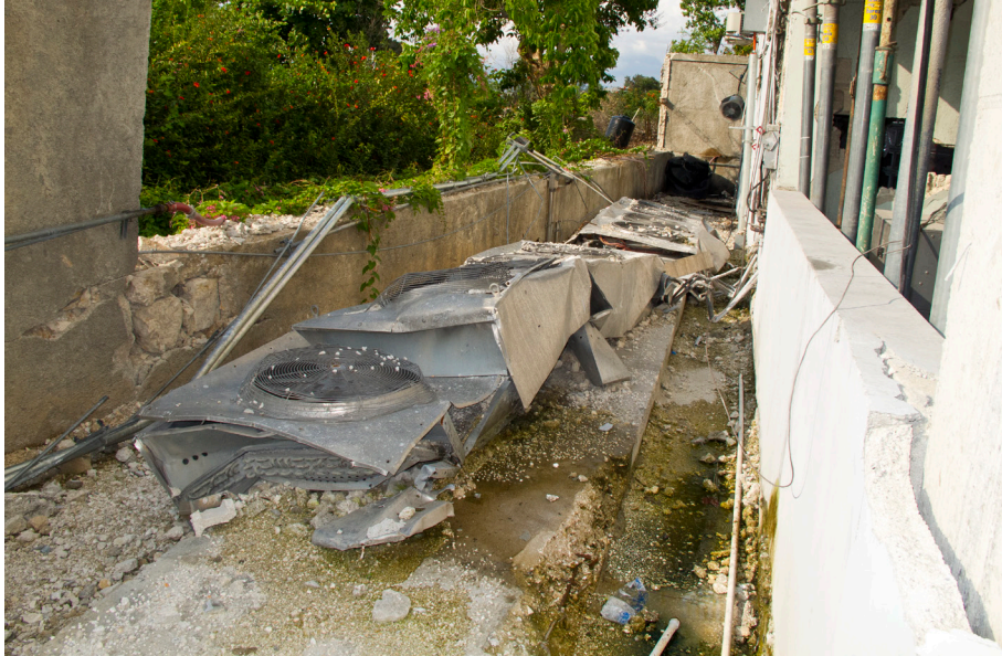
Figure 2-16 Falling debris from security wall and parapet damaged cooling equipment for servers resulting in the data center going off line in the 2011 Haiti earthquake.
