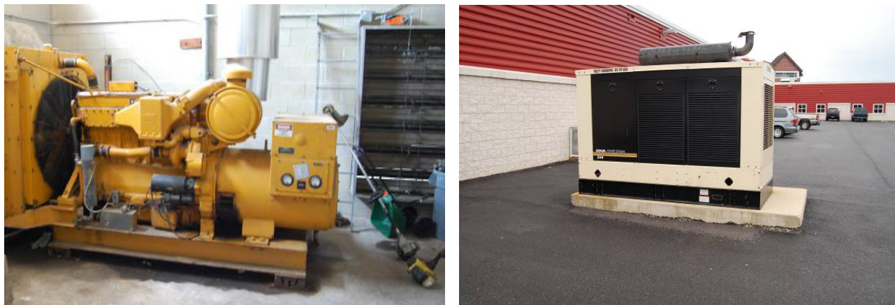
Figure 5-3 Emergency generator installed on the interior (left) and exterior (right).
