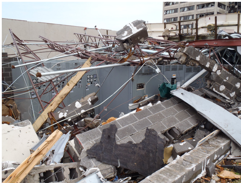
Figure 2-7 Collapsed building housing switchgear and emergency generator after the Joplin, Missouri Tornado (FEMA, 2012a).
