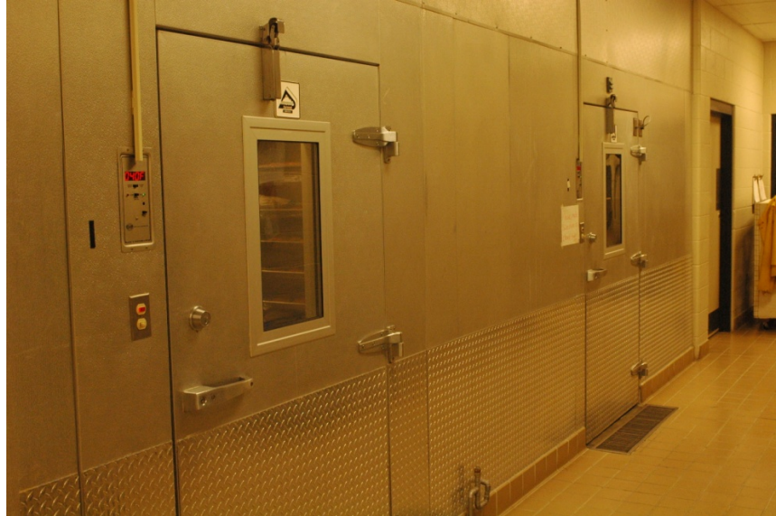
Figure 4-11 Large commercial refrigerator and freezer in commercial kitchen.
