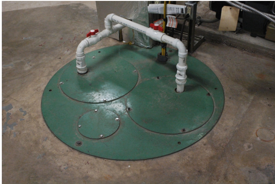
Figure 4-7 Sump cover; pump is within the sump.
