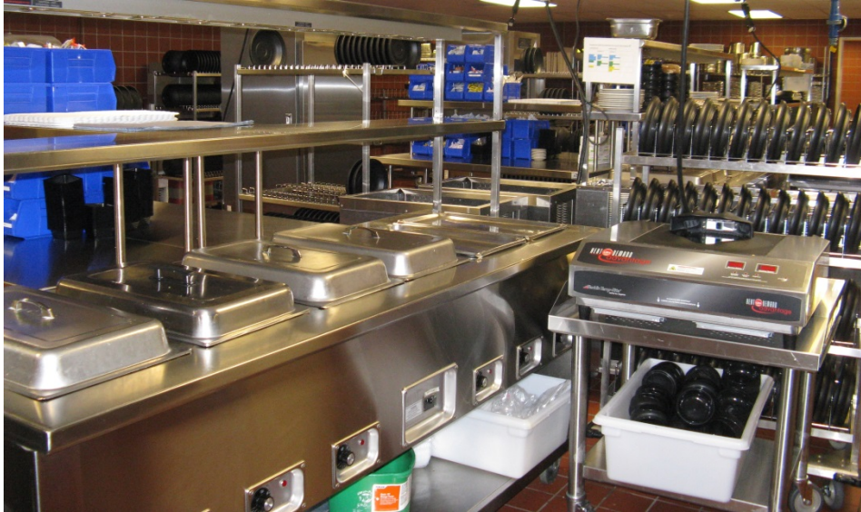
Figure 4-10 Commercial kitchen for critical facility that provides food for occupants.
