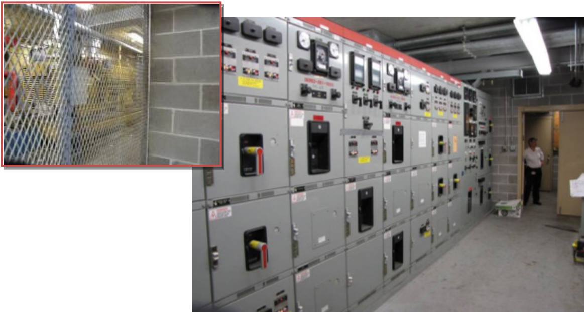
Figure 6-3 Switchgear, normal, and emergency power feeds, and associated equipment elevated to the same level as the emergency generator at UTMB, Galveston, Texas in 2010.
