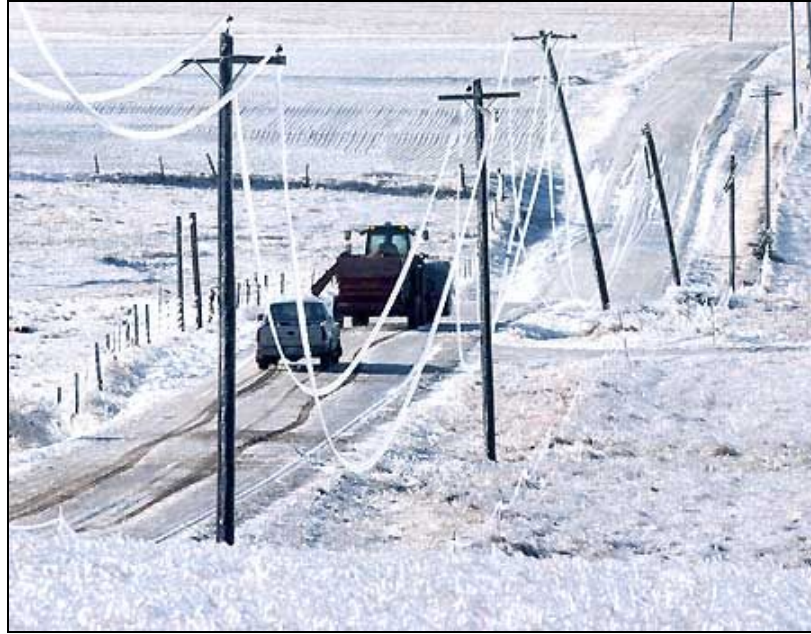
Figure 2-2 Damage to overhead distribution line caused by weight of ice accumulation (Nyether, 2014).
