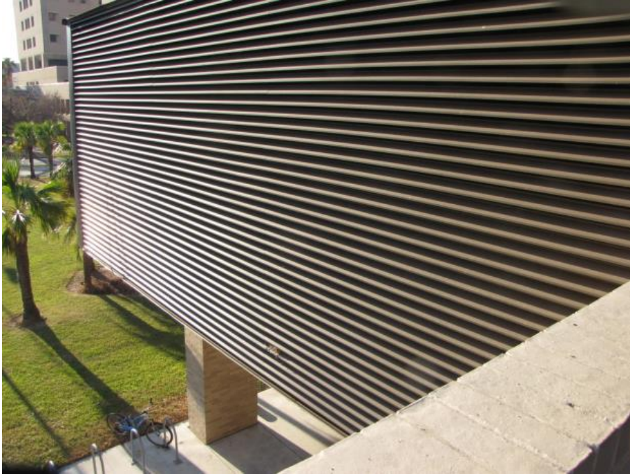
Figure 6-2 Example of an elevated generator; photograph shows the intake louver in Galveston, Texas, 2010.
