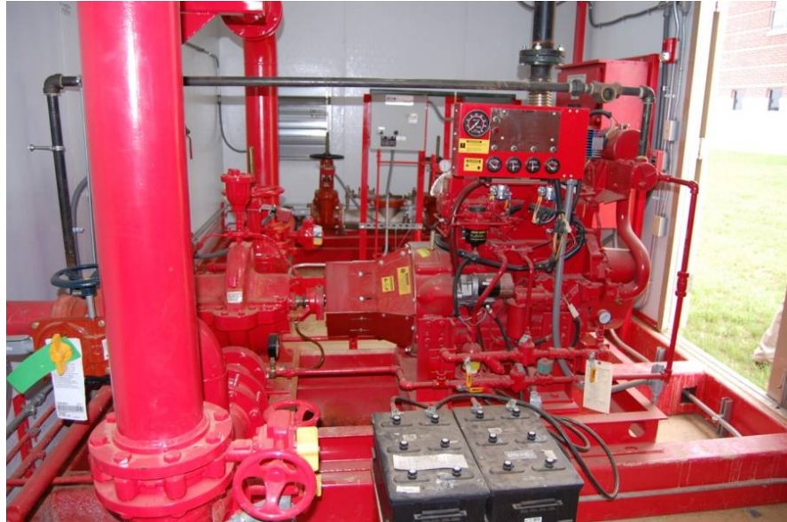
Figure 6-1 Diesel-driven fire pumps.
