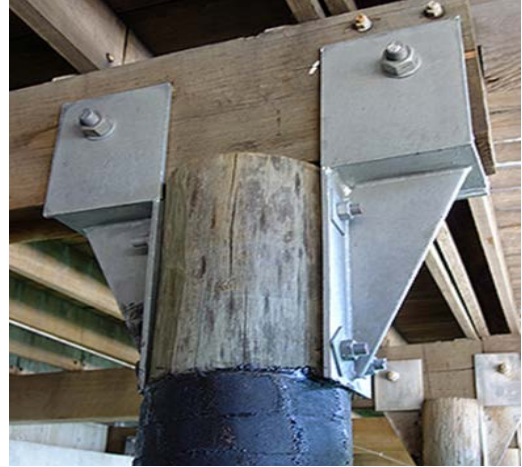
Figure 5.5.4. Reinforce wharves, docks and boardwalks by splicing and reinforcing the structural components of piers and piles (Source: Professional Diving Services, 2020).
