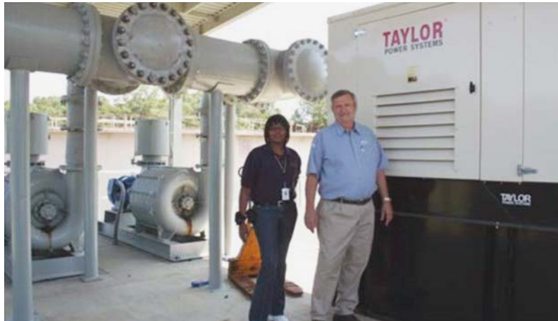
Figure 4.1.3. Installing an emergency backup generator can provide power to help a water treatment plant continue to operate during a flood. (Source: U.S. Environmental Protection Agency [EPA], 2014)
