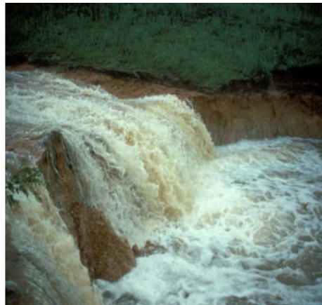
Figure 2.3.11. Headcut erosion could lead to an accidental release from the impoundment. (Source: NRCS, 2017)
