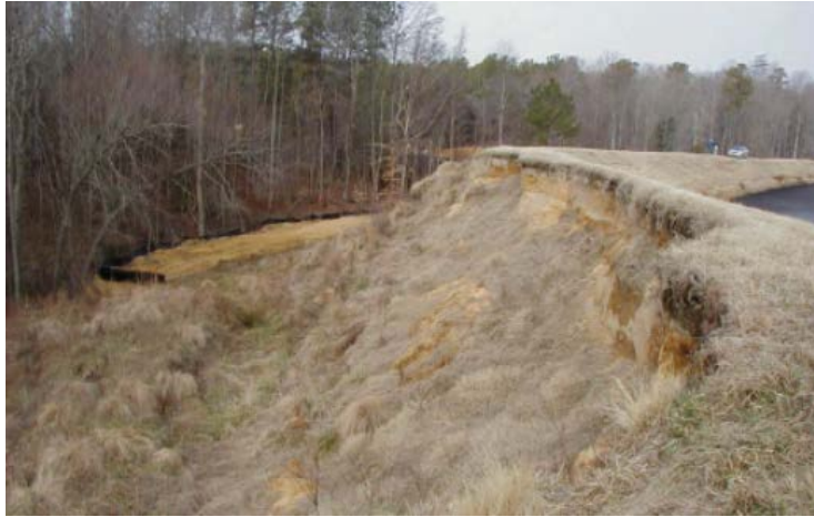
Figure 2.3.3. Example of failed downstream slope. (Source: U.S. Forest Service, 2012)
