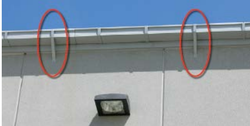
Figure 3.3.2.4. Sheet metal straps (circled) attached to an existing gutter to increase wind uplift resistance.
