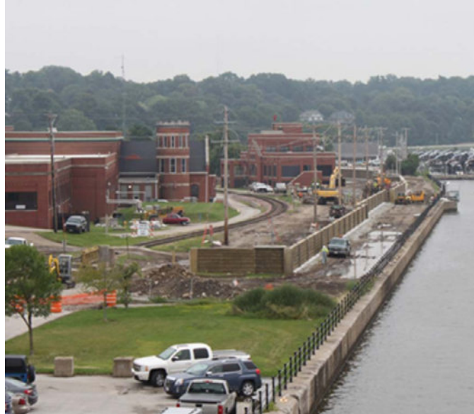
Figure 4.1.2. Constructing a floodwall around a water treatment plant can protect buildings and equipment from flood damage. (Source: U.S. Army Corps of Engineers, 2013)
