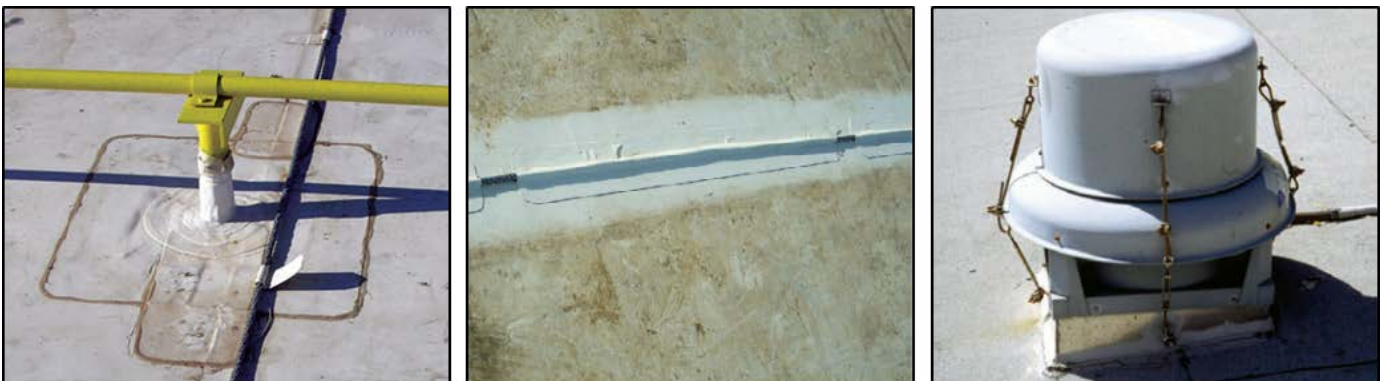
Figure 3.3.2.5. Rooftop periodic gas line supports using a steel angle welded to a pipe that was anchored to the roof deck for lateral and uplift resistance (left). Use of intermittent membrane flashing to secure a lightning protection system conductor (center). Cables attached prevent rooftop equipment cowling from blowing off (right).
