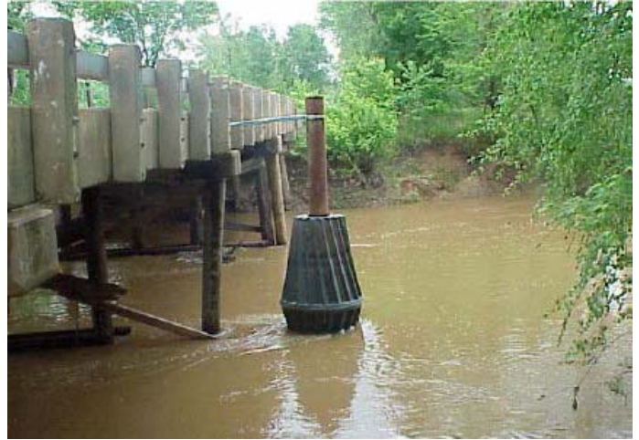
Figure 1.4.20. Pile-mounted debris sweepers can effectively direct debris away from bridge piers (FHWA, 2005).
