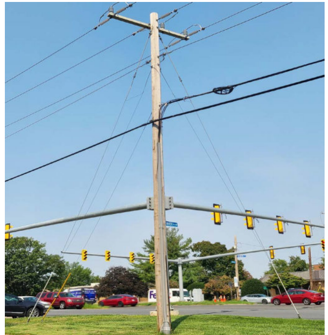
Figure 4.3.5. Typical utility pole with multiple guy wires and anchors.
