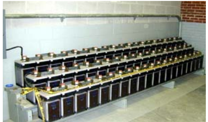
Figure 4.3.10. The existing battery bank can be modified or augmented to provide additional backup power to the substation. (Source: OSHA, No Date)
