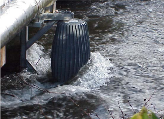
Figure 1.4.19. A debris sweeper can be attached directly to a pier to deflect debris (FHWA, 2005).
