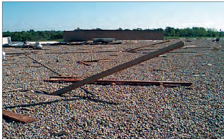
Figure 6-141: A violent tornado showered the roof with missiles (Oklahoma, 1999)
