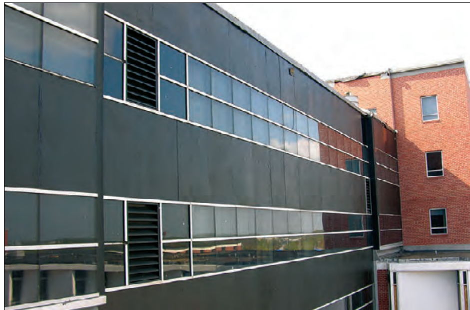
Figure 6-53: Plywood panels (black continuous bands) installed after the glass spandrel panels were broken by roof aggregate. 19 Estimated wind speed: 130 mph. Hurricane Katrina (Mississippi, 2005)
