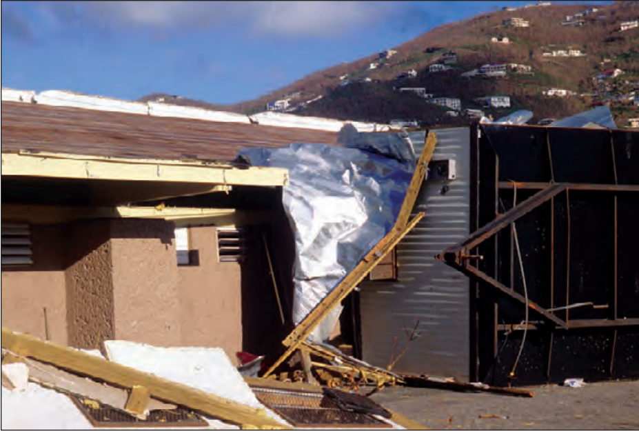
Figure 6-19: This portable classroom was blown up against the main school building. Depending upon the type of exterior wall, an impacting portable classroom may or may not cause wall collapse. Hurricane Marilyn (U.S. Virgin Islands, 1995)
