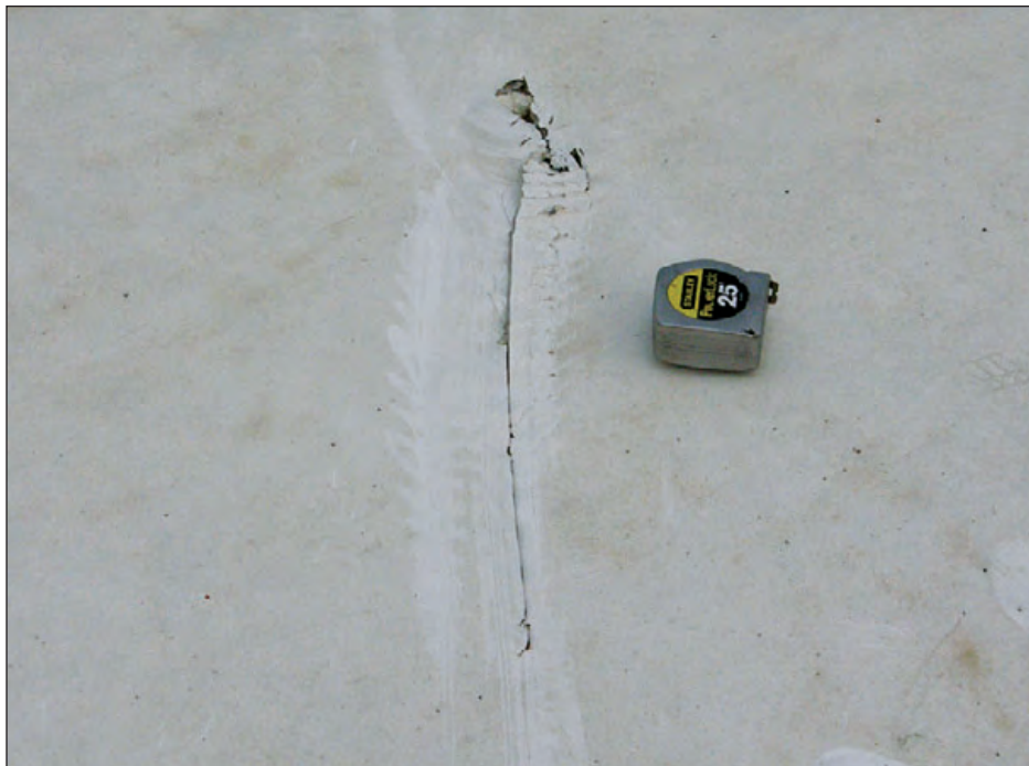
Figure 6-11: The single-ply roof membrane on this school was torn by a missile. The tear was still unprotected 6 days after it was damaged. A substantial amount of water can enter the building through such a tear, unless the deck is water tight (see Figure 6-13) or a secondary roof membrane is used as discussed in Section 6.3.3.7. Estimated wind speed: 105 to 115 mph. Hurricane Ivan (Florida, 2004)
