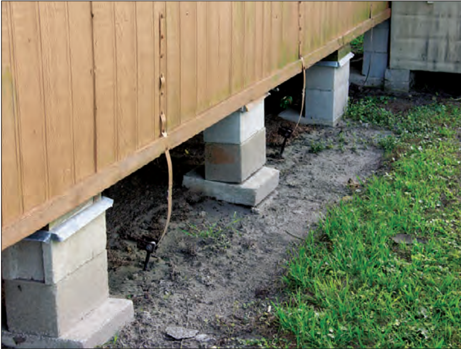
Figure 6-22: The metal straps between this portable classroom and the ground anchors were not taut. This classroom is susceptible to being blown off the piers and to overturning. See Figure 6-27 for a robust anchoring system.
