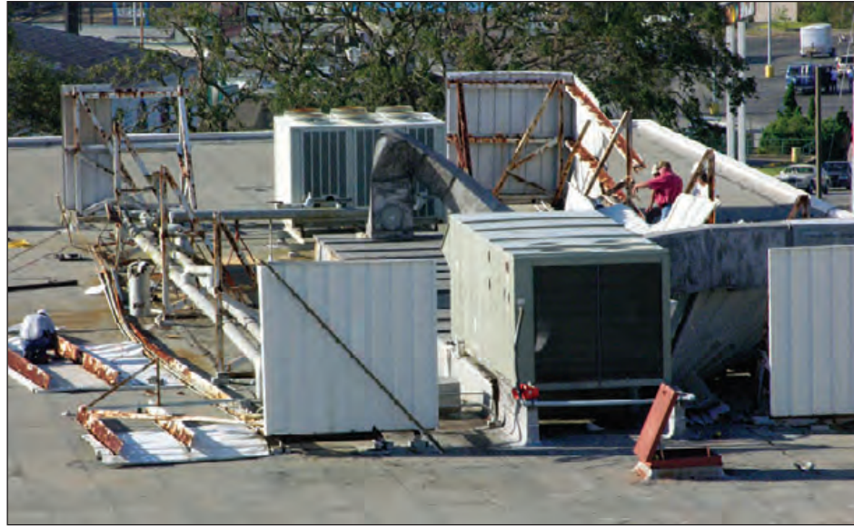
Figure 6-102: Equipment screen panels can puncture roof membranes, break glazing, and cause injury. Estimated wind speed: 105–115 mph. Hurricane Ivan (Florida, 2004)
