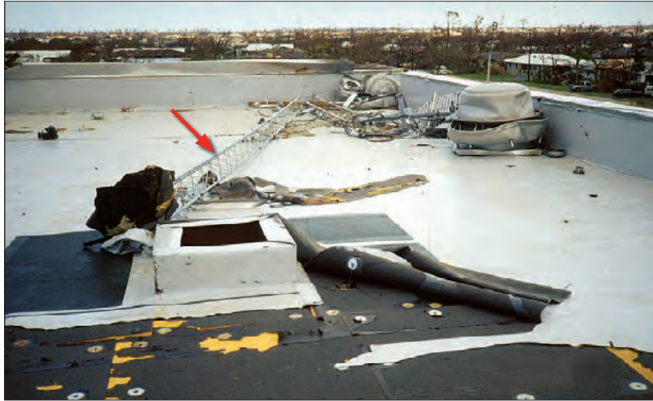
Figure 6-106: The collapse of the antenna tower at this school caused progressive peeling of the roof membrane. Also note that the exhaust fan blew off the curb, but the high parapet kept it from blowing off the roof. Hurricane Andrew (Florida, 1992)
