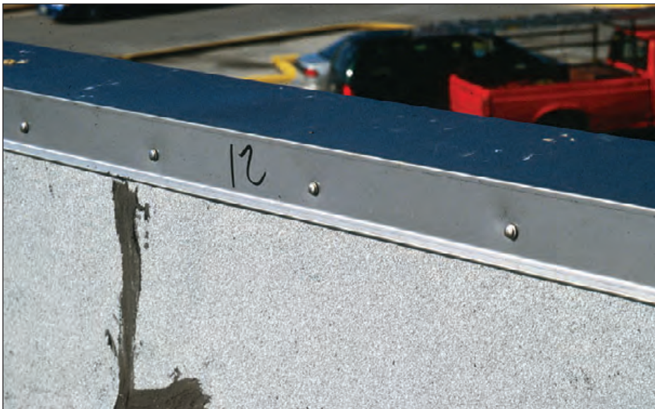
Figure 6-73: Both vertical faces of the coping were attached with exposed fasteners instead of concealed cleats. Typhoon Paka (Guam, 1997)
