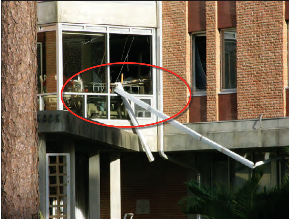
Figure 6-78: Blow-off of this downspout resulted in glazing breakage. Estimated wind speed: 105–115 mph. Hurricane Ivan (Florida, 2004)
