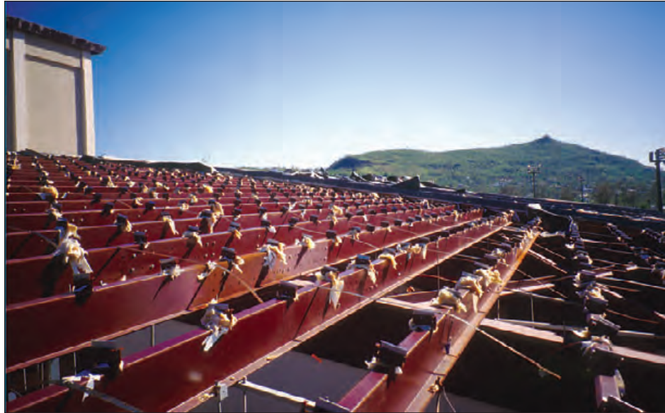
Figure 6-20: This newly-constructed gymnasium had a structural metal roof panel (3-inch trapezoidal ribs at 24 inches on center) applied over metal purlins. The panels detached from their concealed clips. A massive quantity of water entered the school and buckled the wood gym floor. Typhoon Paka (Guam, 1997)
