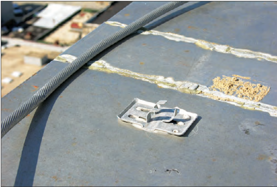
Figure 6-111: This conductor connector was adhered to the coping. The conductor deformed the connector prongs under wind pressure, and pulled away from the connector. Estimated wind speed: 130 mph. Hurricane Katrina (Mississippi, 2005)
