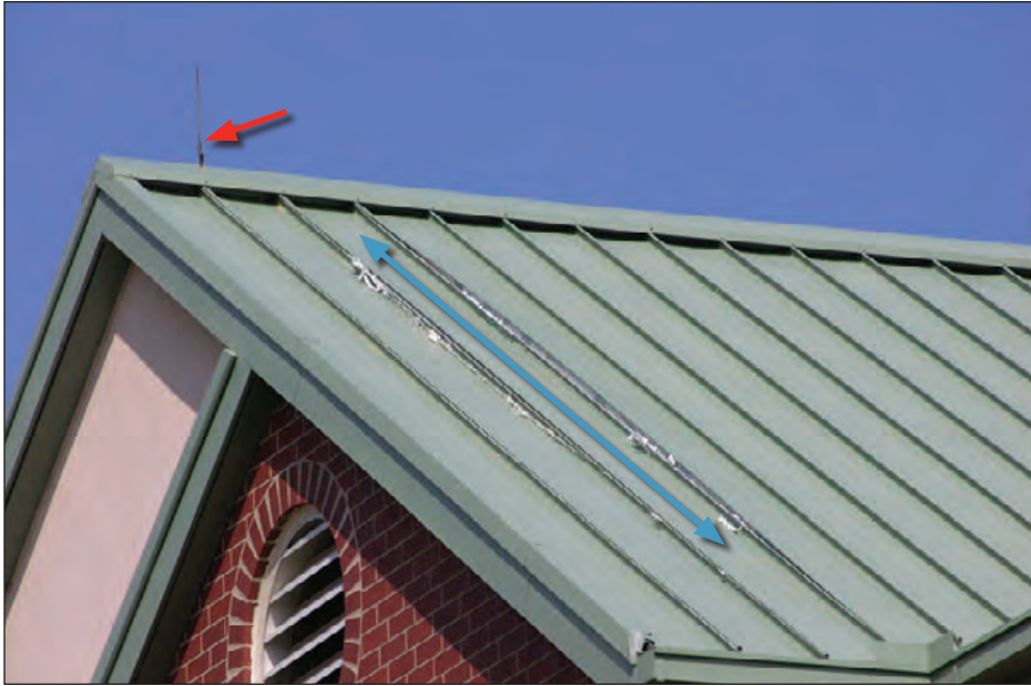
Figure 6-67: Three of the panel ribs opened up (one to the right of the blue arrow and two to the left). The LPS conductor serving the air terminal (red arrow) ran underneath the ridge flashing. Estimated wind speed: 105–115 mph. Hurricane Ivan (Florida, 2004)
