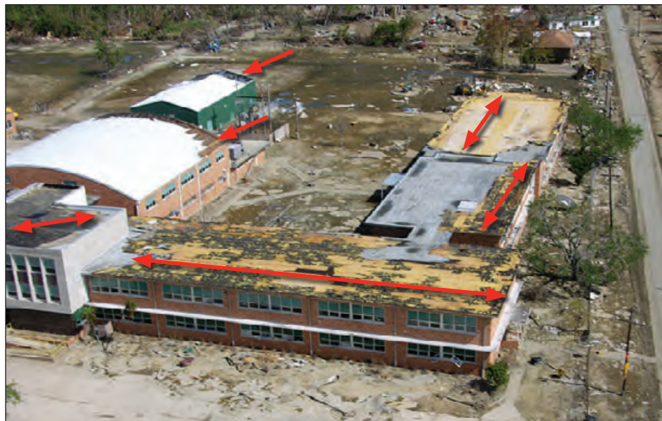
Figure 6-1: Large portions of the roof coverings blew off of this school. Estimated wind speed: Approximately 125 to 130 miles per hour (mph). 2 Hurricane Katrina (Louisiana, 2005)
