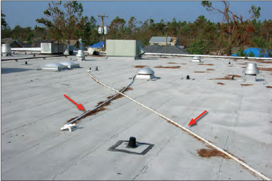
Figure 6-101: These two condensate drain lines detached from their HVAC units. They had not been anchored to the roof. Estimated wind speed: 125 mph. Hurricane Katrina (Mississippi, 2005)
