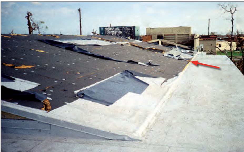
Figure 6-85: This mechanically attached single-ply membrane progressively tore after being cut by wind-borne debris. Hurricane Andrew (Florida, 1992)
