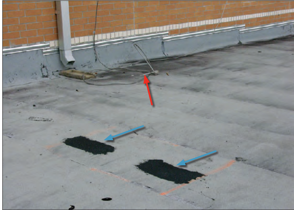
Figure 6-109: An air terminal (red arrow) debonded from the roof. Even though the school had a tough membrane (modified bitumen), the displaced air terminal punctured the membrane in two locations (blue arrows). Hurricane Charley (Florida, 2004)
