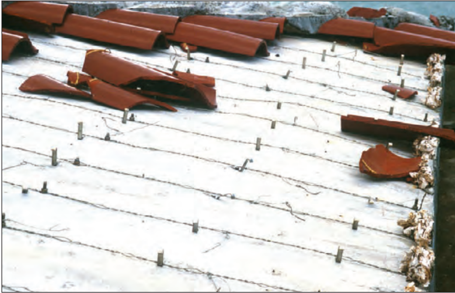
Figure 6-84 These wire-tied tiles were installed over a concrete deck. The failure was attributed to lack of vertical restraint, which allowed the tiles to lift and then be broken when they slammed back down onto the deck. Typhoon Paka (Guam, 1997)
