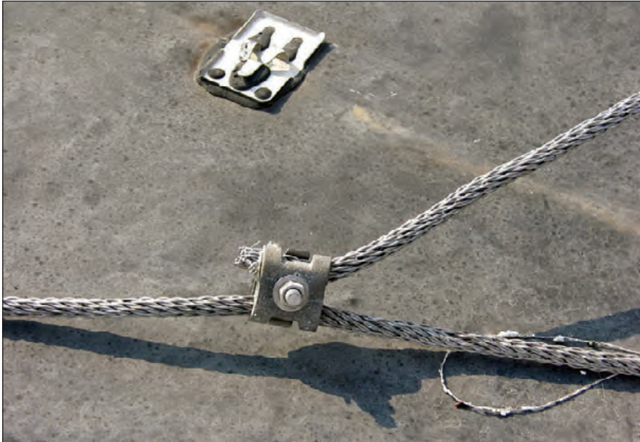
Figure 6-117: Bolted splice connectors are recommended to prevent free ends of connectors from being whipped around by wind. Estimated wind speed: 130 mph. Hurricane Katrina (Mississippi, 2005)
