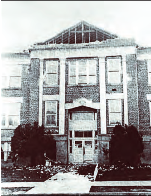
Figure 4-19: The student body president was killed here by falling brickwork, Seattle, WA, 1949
