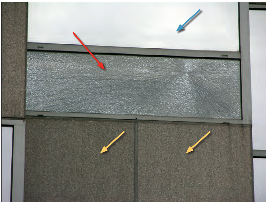
Figure 6-54: The red arrow shows a piece of laminated glass that was broken, but remained in the frame to protect the building's interior. The blue arrow shows unbroken laminated glass. The yellow arrows show granite wall panels. Estimated wind speed: 105 mph. Hurricane Katrina (Louisiana, 2005)
