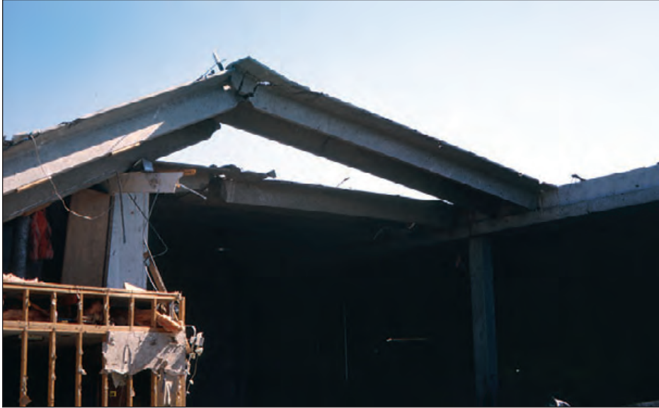
Figure 6-40: Twin-Tee roof panel lifted as a result of the combined effects of wind uplift and pre-tension. Tornado (Missouri, May 2003)
