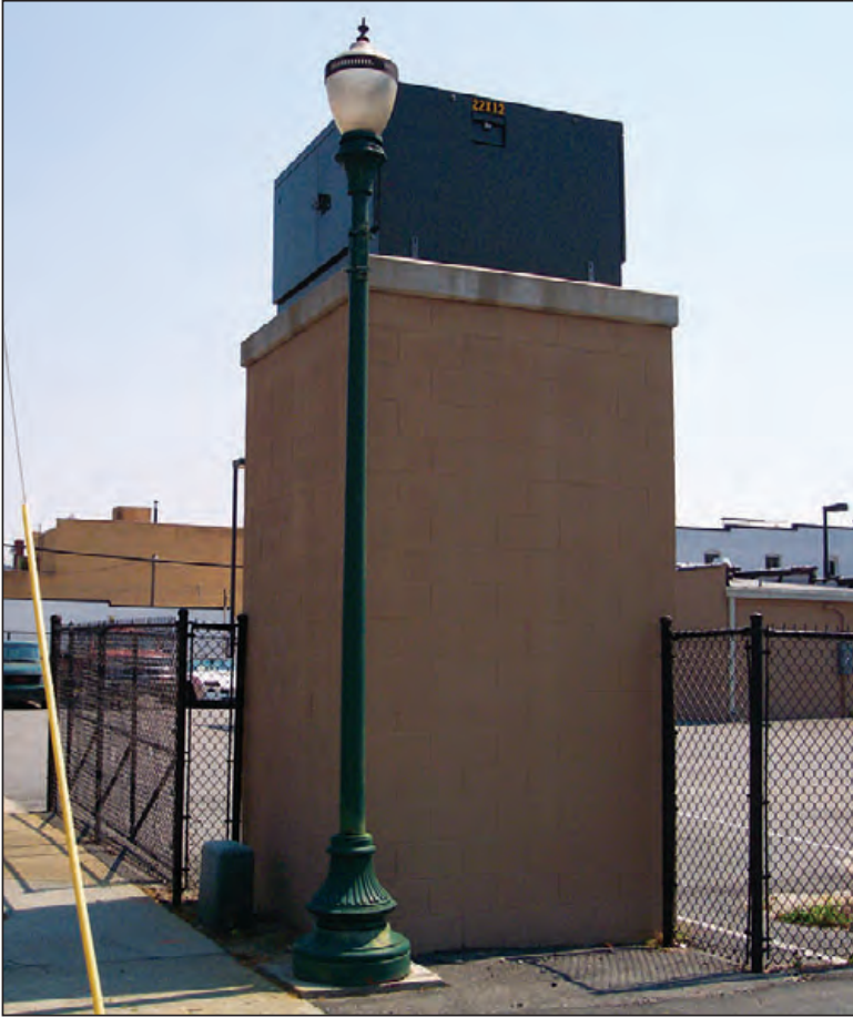
Figure 5-30: Utility component elevated above flood level
