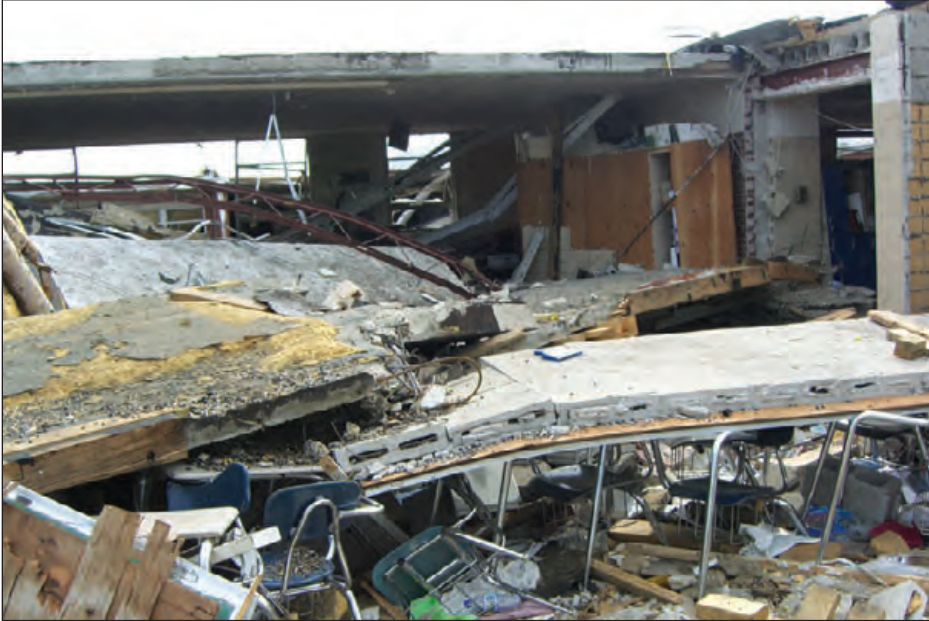
Figure 6-143 : Unreinforced masonry walls and hollow-core concrete roof planks collapsed. Enterprise Tornado (Alabama, 2007)
