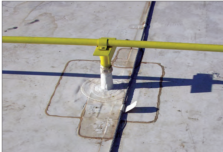
Figure 6-100: At a periodic gas line support on this roof, a steel angle was welded to a pipe that was anchored to the roof deck. A strap looped over the gas line and was bolted to the support angle. Such a connection provides resistance to lateral and uplift loads.
