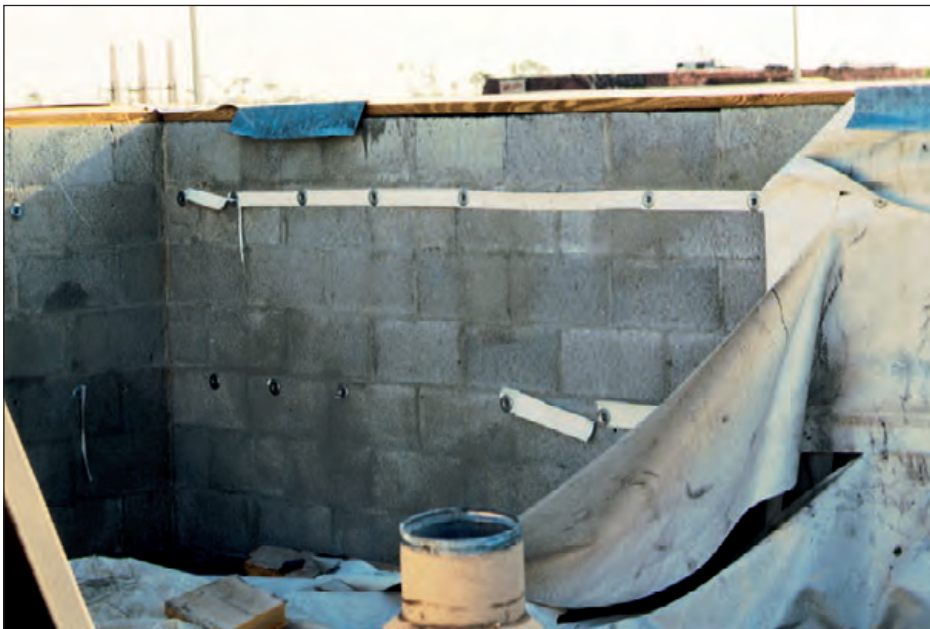
Figure 6-79: If mechanically attached base flashings have an insufficient number of fasteners, the base flashing can be blown away. Hurricane Andrew (Florida, 2004)
