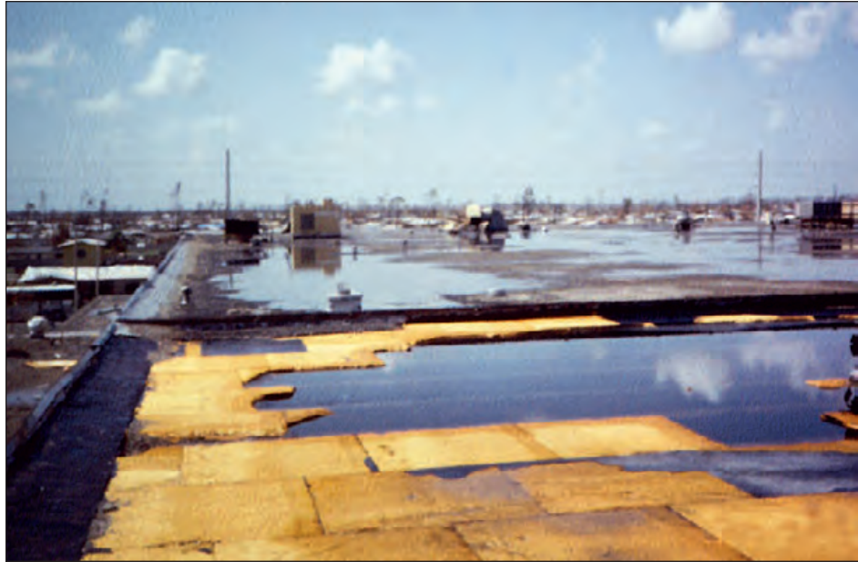
Figure 6-13: Extensive roof covering and rooftop equipment damage occurred on this school. However, the cast-in-place concrete deck kept most of the water from entering the school. Hurricane Andrew (Florida, 1992)
