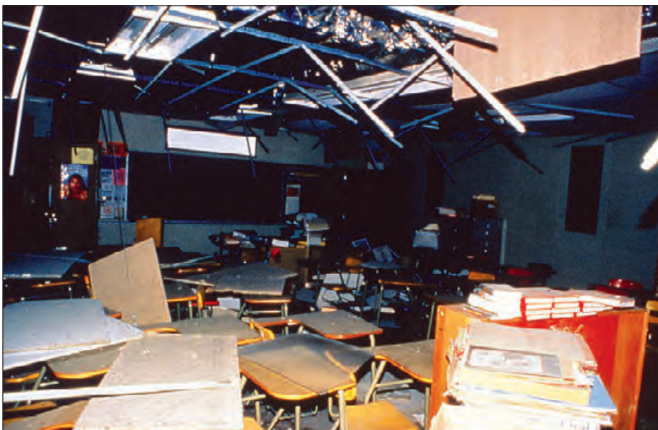
Figure 4-25: Ceiling damage, Northridge, CA, 1994
