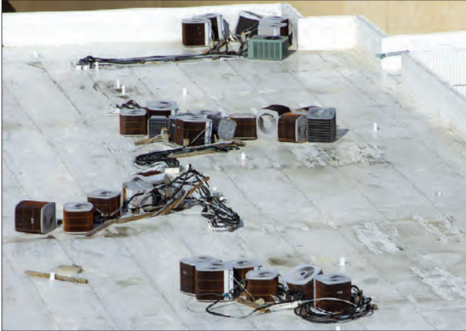
Figure 6-94: These condensers were blown off their sleepers. Displaced condensers can rupture roof membranes and refrigerant lines. Estimated wind speed: 120 mph. Hurricane Katrina (Mississippi)
