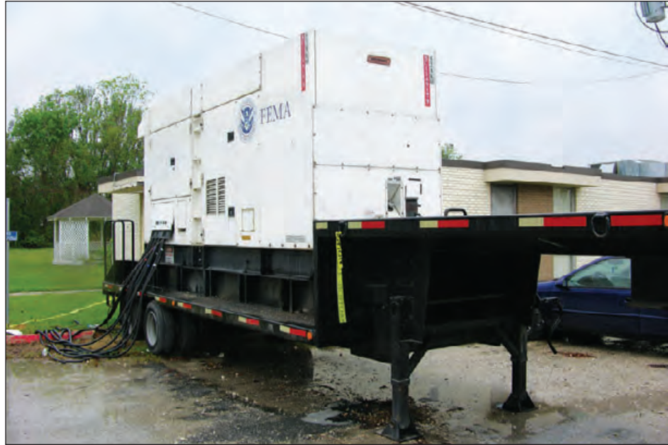
Figure 6-118: In lieu of permanent on-site emergency generators, portable generators can be an economical way to provide electrical power to schools used as hurricane recovery centers. Estimated wind speed: 108 mph. Hurricane Ike (Texas, 2008)
