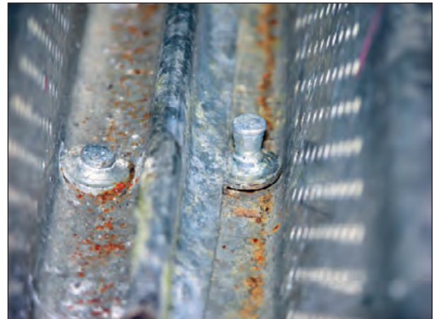
Figure 6-38: View looking along a sidelap of a deck attached with powder-driven pins. The right pin does not provide adequate uplift and shear resistance.
