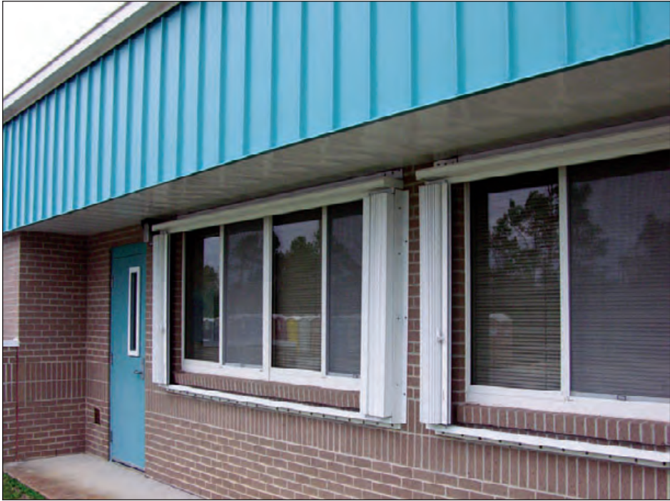
Figure 6-125: This school has accordion shutters. Estimated wind speed: 105–115 mph. Hurricane Ivan (Florida, 2004)
