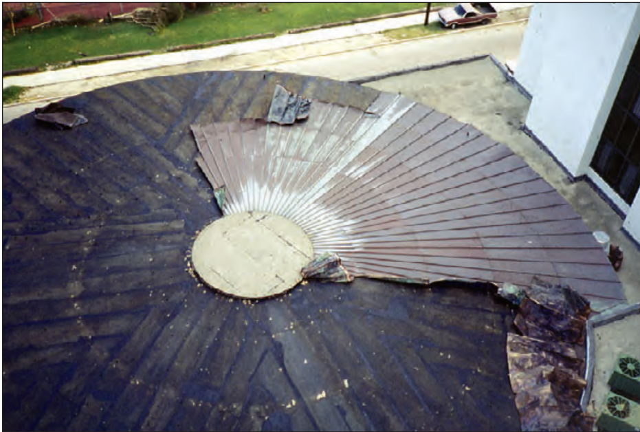
Figure 6-80: The secondary membrane prevented significant leakage into the building after the copper roof blew off. Hurricane Andrew (Florida, 1992)
