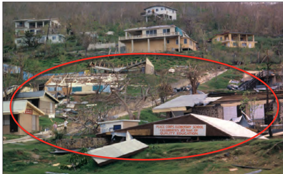
Figure 6-18: This elementary school was composed of several buildings. The building in the foreground collapsed and several others experienced significant structural damage. The buildings further up the hillside are residences. Hurricane Marilyn (U.S. Virgin Islands, 1995)
