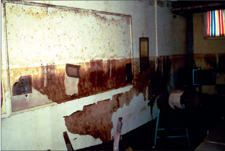
Figure 5-18: Saturation damage extends above the water line in this grade school in Gurnee, IL.
