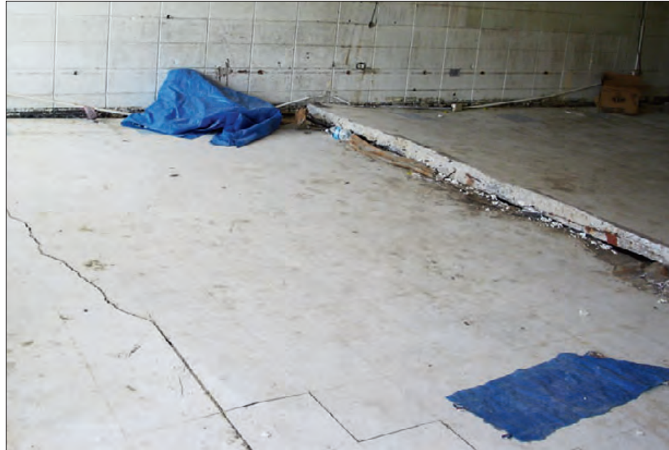
Figure 5-15: Concrete slab ruptured by hydrostatic pressure (buoyancy) induced by the floodwaters of Hurricane Katrina (2005)
