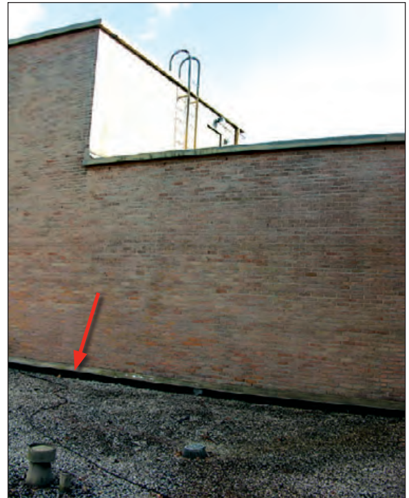
Figure 6-59: Water leaked inside along the base of the brick veneer walls (red arrow). Estimated wind speed: 115 mph. Hurricane Katrina (Louisiana, 2005)
