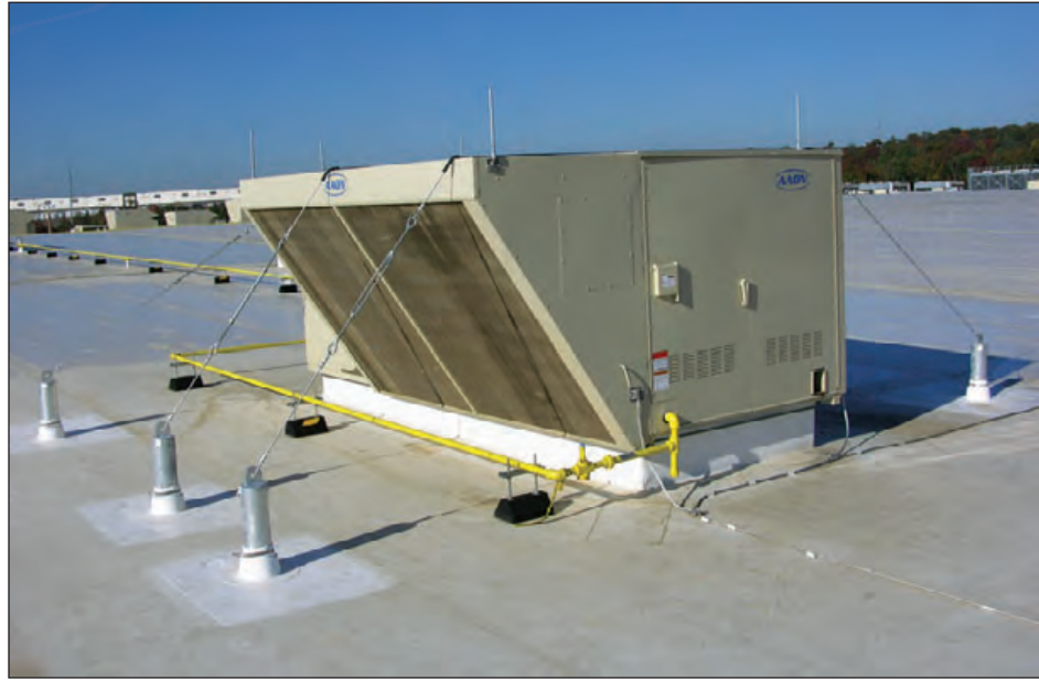
Figure 6-135: To strengthen attachment of this HVAC unit, robust pipe anchors were attached to the deck and cables with turnbuckles installed.
