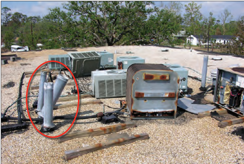
Figure 6-137: These condensers were simply mounted on wood sleepers that rested on the roof surface. Note the damaged exhaust stacks and missing rain caps (red oval). Estimated wind speed: 105 mph. Hurricane Katrina (Mississippi, 2005)
