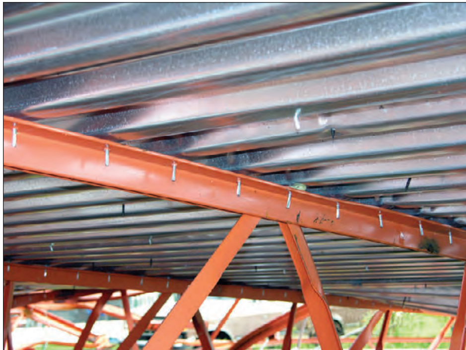
Figure 6-35: Even though the roof structure blew off, because of the strength and reliability of the screwed deck connections, the decking remained attached to the joists. Hurricane Charley (Florida, 2004)
