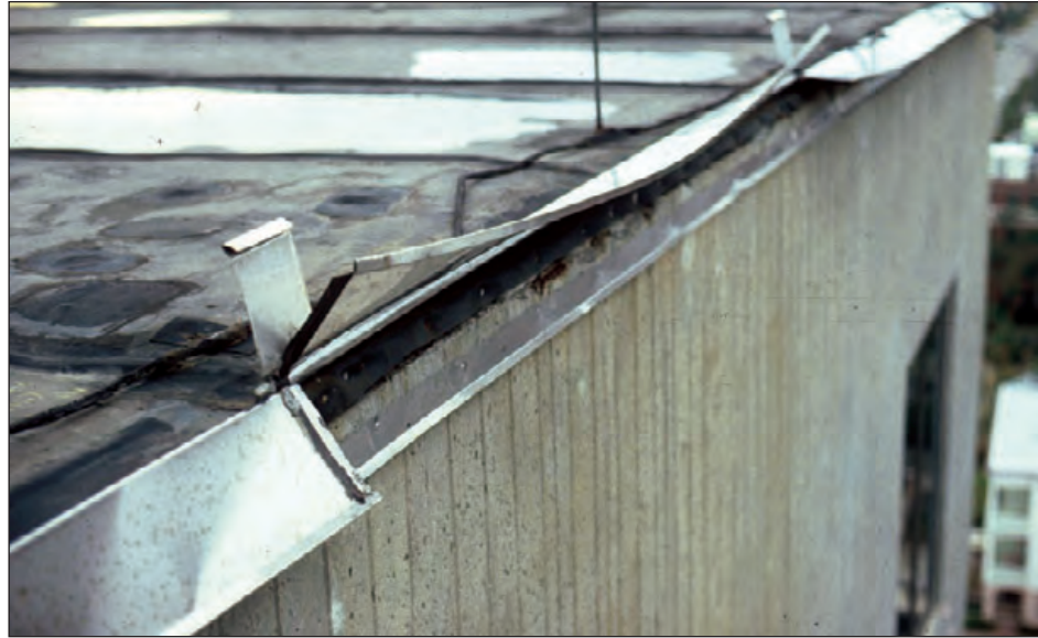
Figure 6-71: The metal edge flashing on this building disengaged from the continuous cleat and the vertical flange lifted. Hurricane Hugo (South Carolina, 1989)
