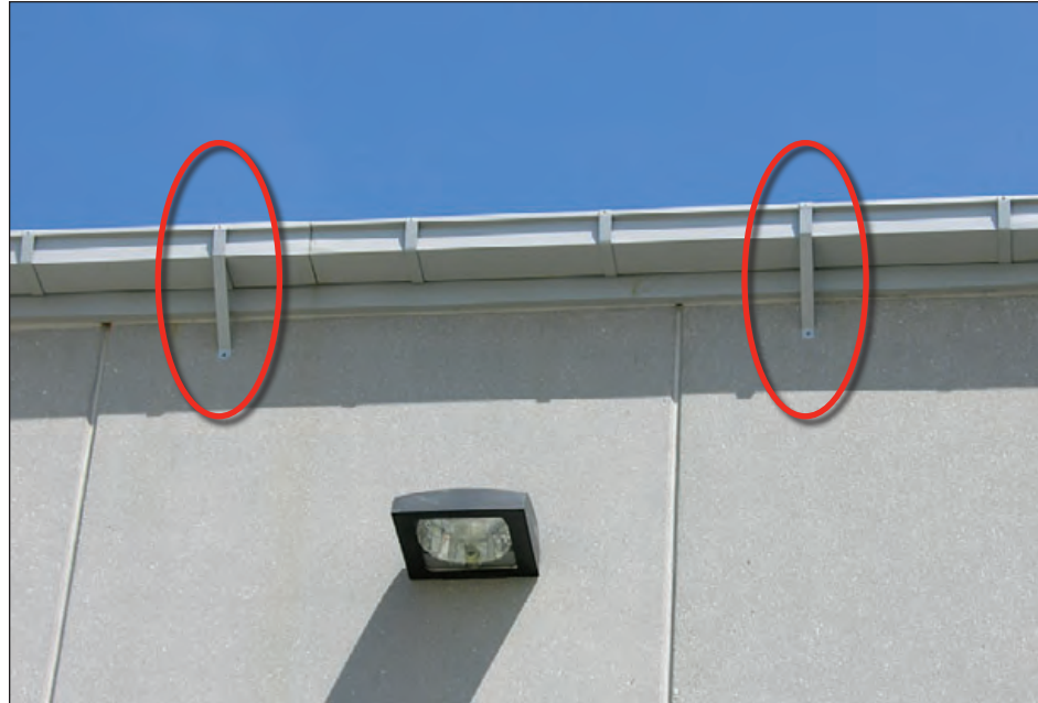
Figure 6-77: Sheet metal straps were attached to an existing gutter that lacked sufficient uplift resistance.
