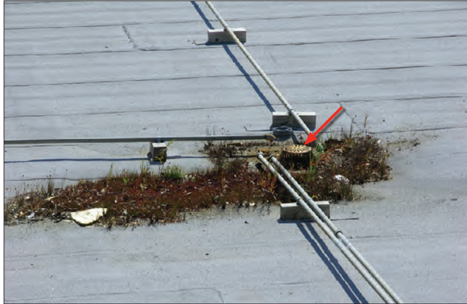
Figure 6-32: Dirt and vegetation surrounded this roof drain (red arrow) and impeded drainage. Roof drains should be checked at least annually and cleaned of debris if found. Drains should also be checked prior to hurricane landfall. Hurricane Ike (Texas, 2008)
