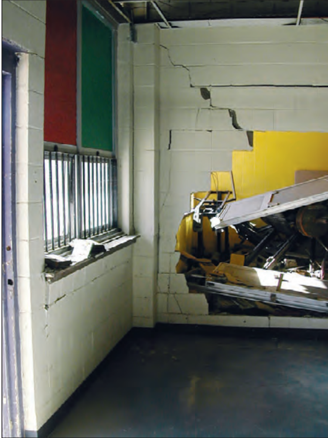
Figure 5-14: Interior unreinforced masonry walls of the Port Sulphur High School in Louisiana were damaged by hydrostatic loads associated with Hurricane Katrina's storm surge (2005)
