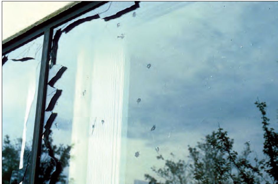
Figure 6-14: The outer window panes were broken by aggregate from a built-up roof. Estimated wind speed: 104 mph. Hurricane Hugo (South Carolina, 1989)
