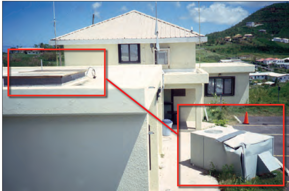
Figure 6-25: Lack of fasteners resulted in blow-off of the HVAC unit, which caused extensive interior water damage and interrupted facility use. Hurricane Marilyn (U.S. Virgin Islands, 1995)
