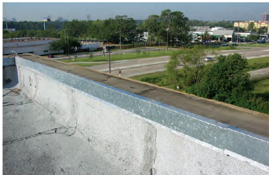
Figure 6-72: The coping blew off because of inadequate attachment of the cleats. Estimated wind speed: 92 mph. Hurricane Ike (Texas, 2008)
