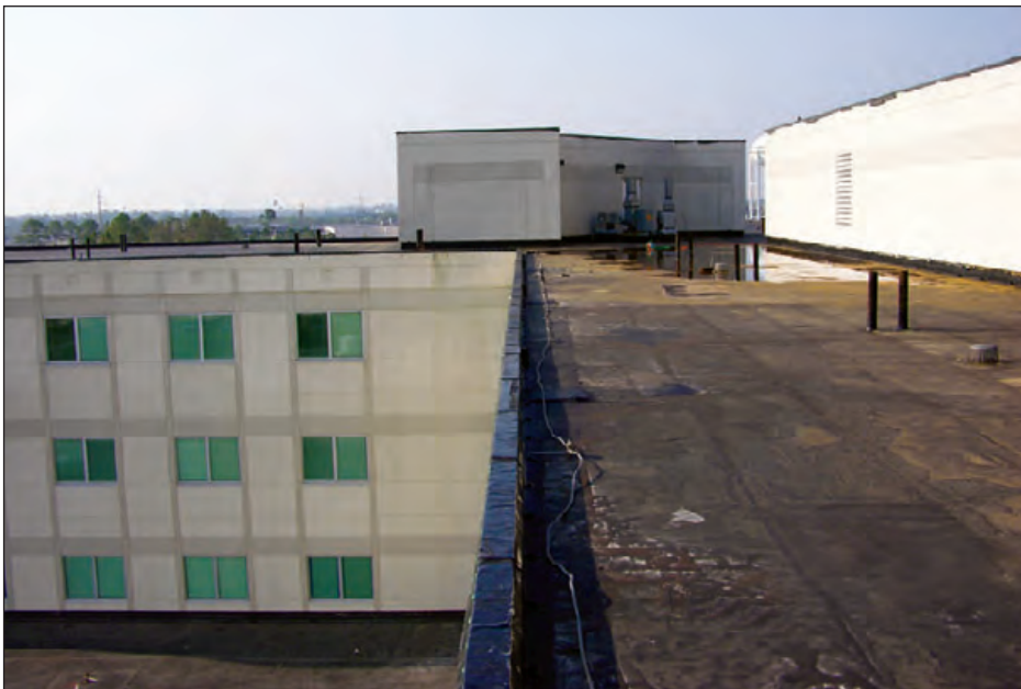
Figure 6-120: The roof and a portion of the EIFS on this 5-year-old building blew off. Water leaked into the floor below. The floor was taken out of service for more than a month. Estimated wind speed: 130 mph. Hurricane Katrina (Mississippi, 2005)
