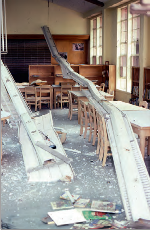
Figure 4-10: Fallen light fixtures, library, Coalinga, CA, 1983
