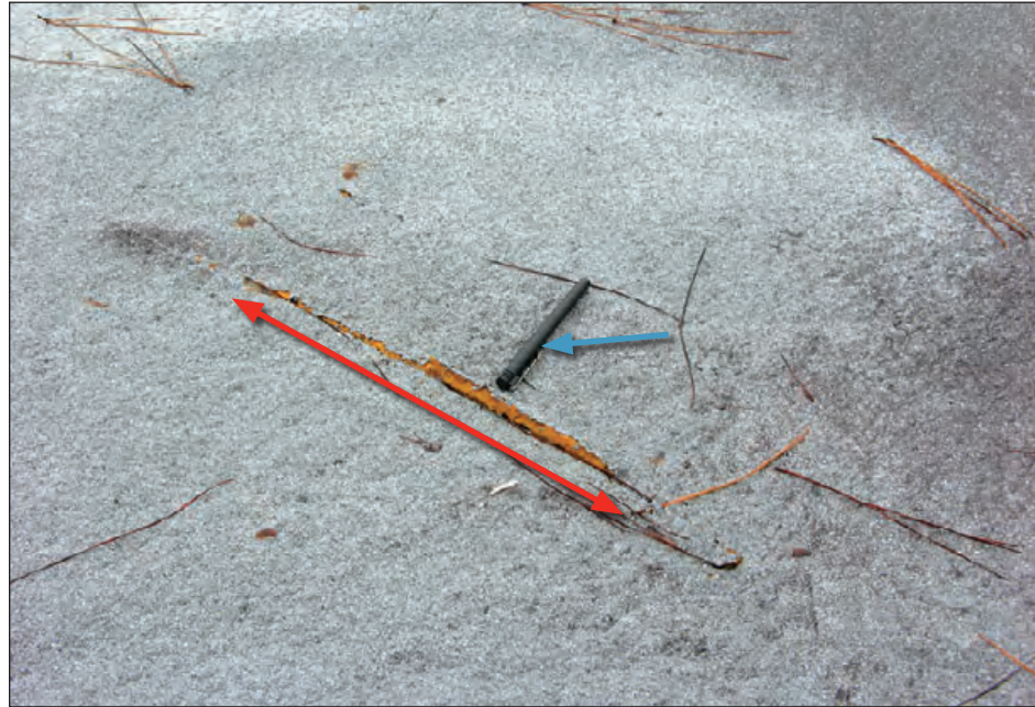
Figure 6-81: Although a missile cut into the SPF, the roof was still watertight. The ink pen (blue arrow) shows the relative size of the impact area. Estimated wind speed: 110 mph. Hurricane Ike (Texas, 2008)
