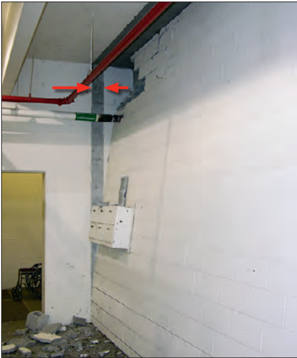
Figure 6-56: The red arrows show the original location of a CMU wall that nearly collapsed following a rolling door failure. Estimated wind speed: 140–160 mph. Hurricane Charley (Florida, 2004)
