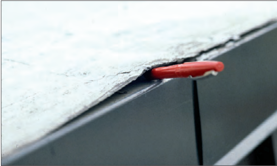
Figure 6-70: The ink pen shows an opening that the wind can catch to cause lifting and peeling of the membrane.
