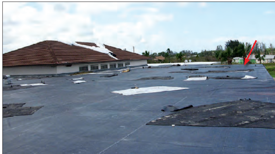
Figure 6-75: The original modified bitumen membrane was blown away after the gutter lifted in the area shown by the red arrow (the black membrane is a temporary roof). Hurricane Francis (Florida, 2004)
