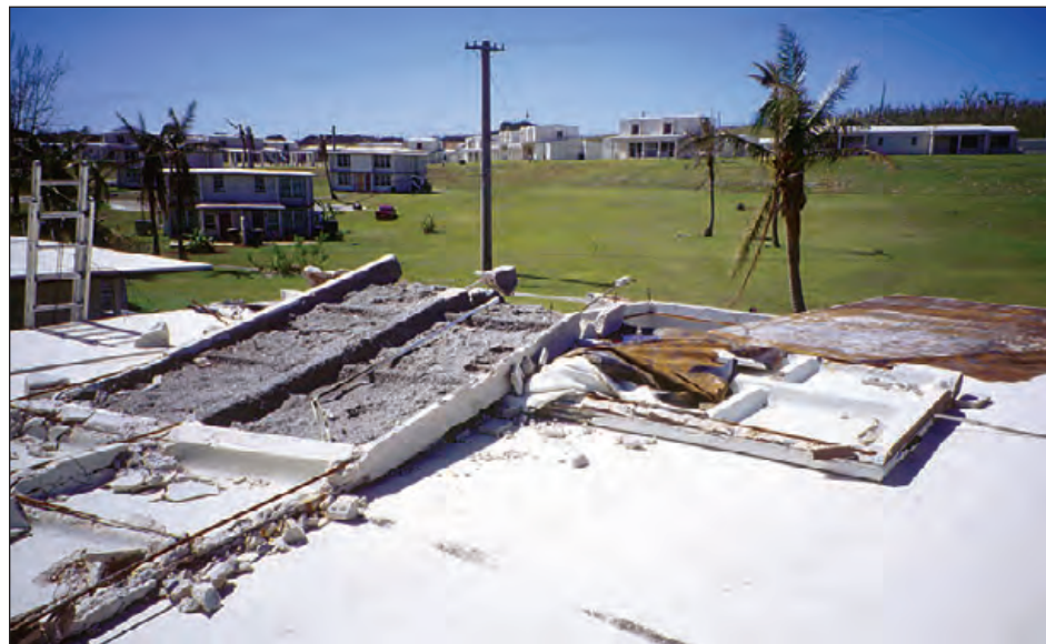
Figure 6-39: Portions of this waffled precast concrete roof deck were blown off. Typhoon Paka (Guam, 1997)
