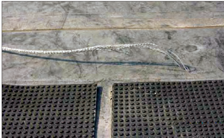
Figure 6-110: View of an end of a conductor that became disconnected. Estimated wind speed: 130 mph. Hurricane Katrina (Mississippi, 2005)
