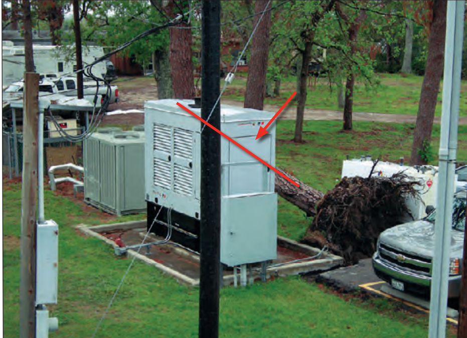
Figure 6-119: The tree shown by the red line nearly fell on the emergency generator (red arrow). Estimated wind speed: 110 mph. Hurricane Ike (Texas, 2008)
