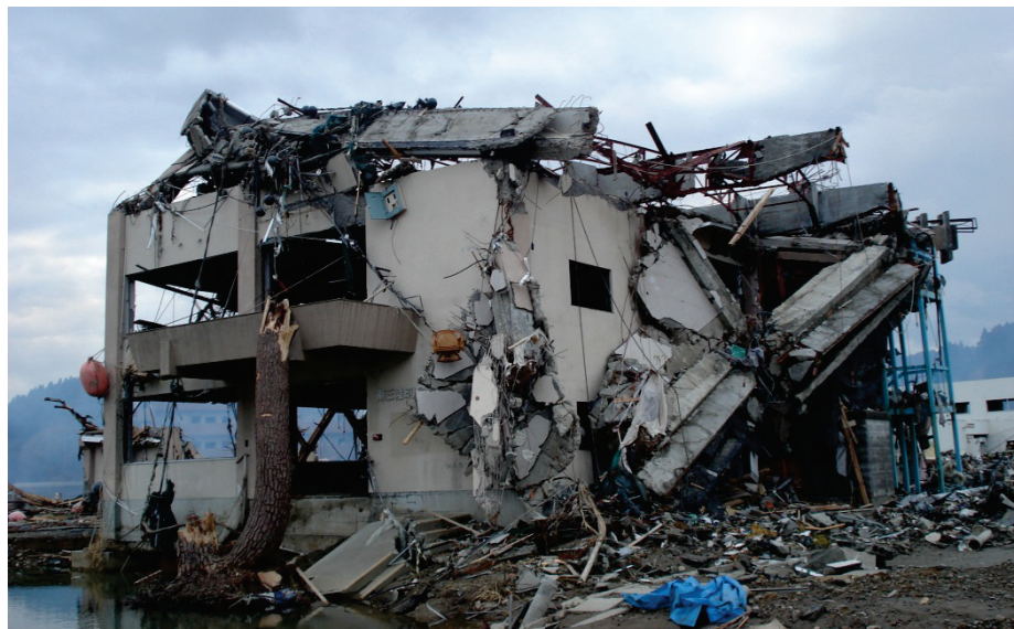
Figure 2-27 Collapsed upper story of reinforced concrete building with steel truss roof, 2011 Tohoku tsunami (photo courtesy of I. Nistor and ASCE, from Chock, et al., 2013b).
