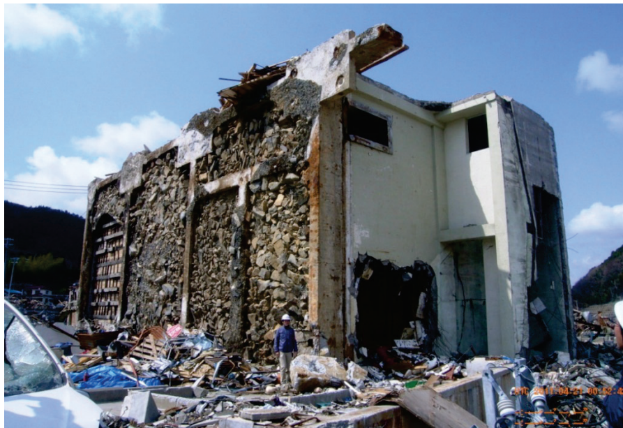
Figure 2-28 Overturned cold storage building in Onagawa, Japan, 2011 Tohoku tsunami (photo courtesy of G. Chock and ASCE, from Chock, et al., 2013b).
