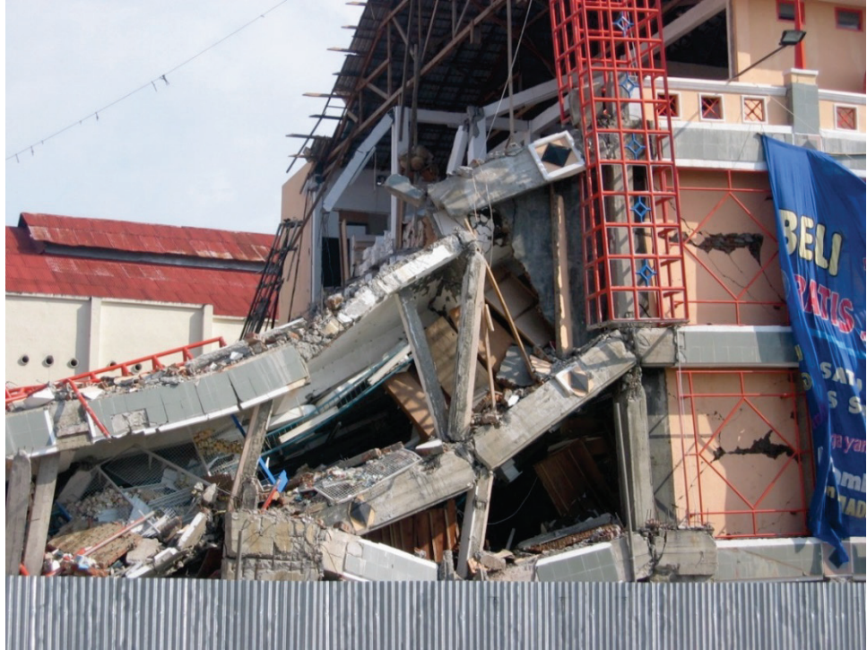
(a) Beam-column connection failures
