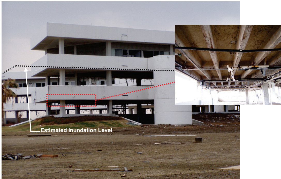
Figure 2-31 Office building in Pass Christian, Mississippi, with a cast-in-place concrete pan joist floor system that suffered nonstructural damage in the first two stories, but no structural damage, 2005 Hurricane Katrina (photos courtesy of I. Robertson).
