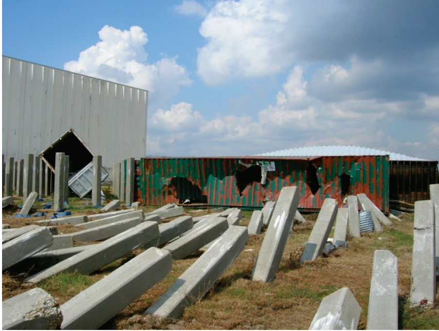
Figure 2-33 Failure of prestressed piles due to damming effect of shipping container, 2005 Hurricane Katrina (photo courtesy of I. Robertson).
