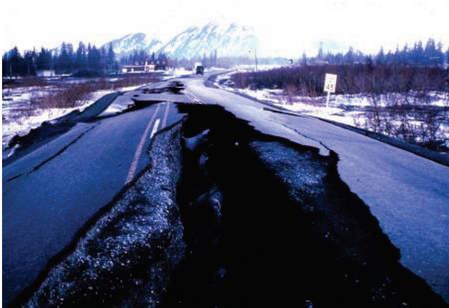
Figure 6-3 Roadway damage as a result of the 1964 Alaska earthquake (photo courtesy of the U.S. Geological Survey).
