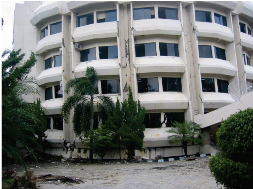
(b) Soft story failure
