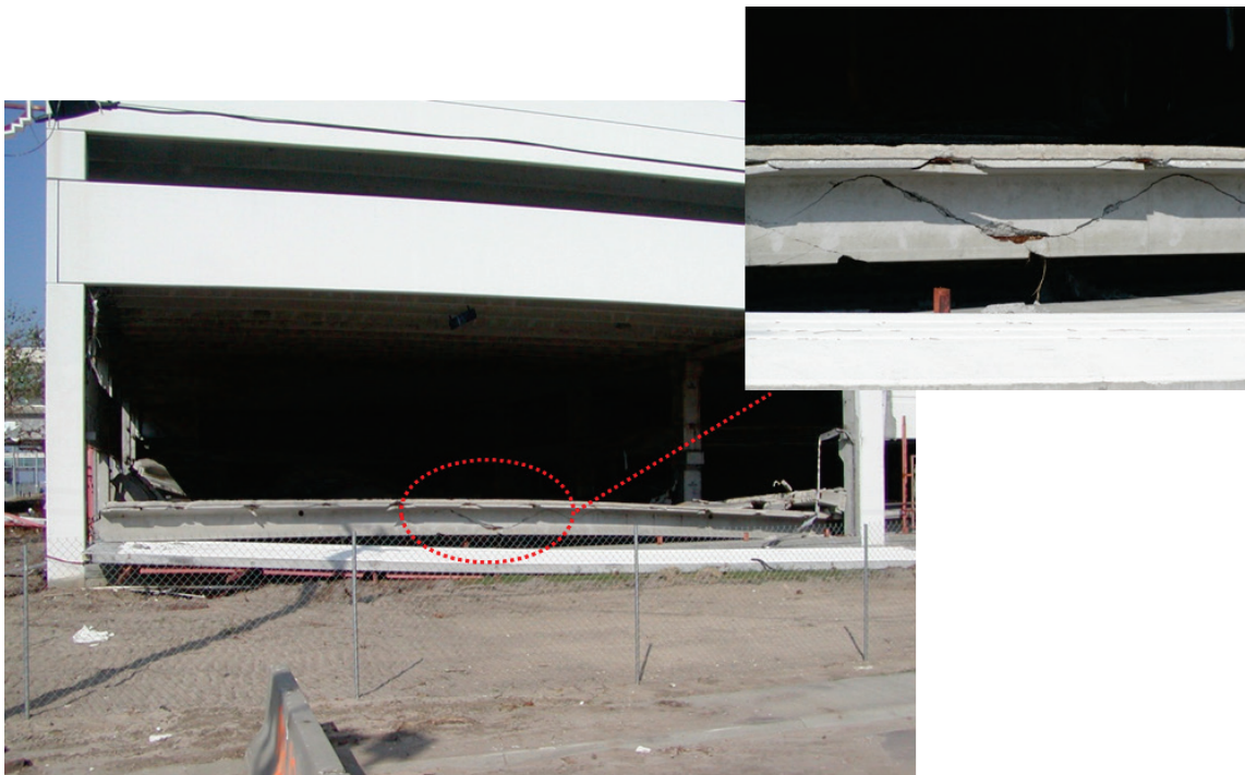
Figure 2-34 Negative bending failure of a prestressed double-tee floor system due to uplift forces, 2005 Hurricane Katrina (photos courtesy of I. Robertson).
