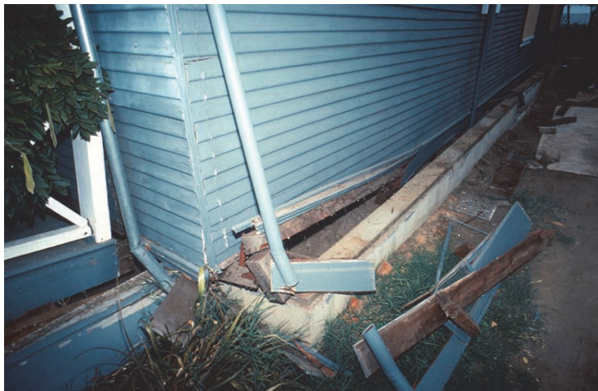
Figure 4-6 House that fell off its foundation in the 1989 Loma Prieta Earthquake.
