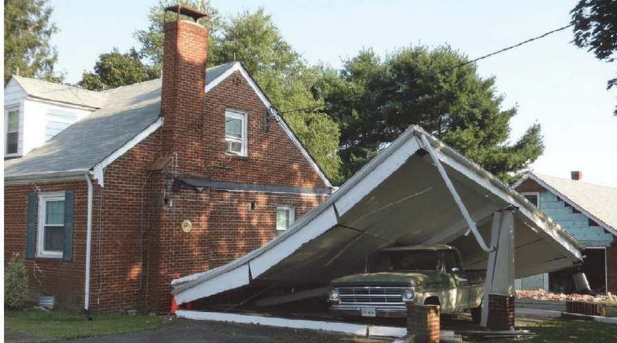
Figure 4-5 This carport, originally supported by but not firmly attached to the adjacent house, became detached from the house during ground shaking (from FEMA P-530).
