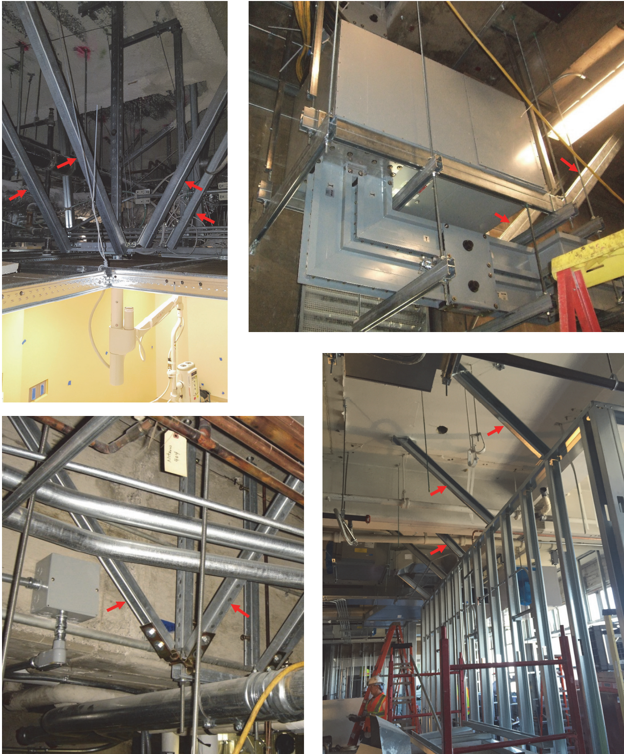
Figure 9-2 Examples of nonstructural bracing. Top left: Ceiling-mounted medical device. Top right: Above-ceiling air handling unit (from FEMA E-74). Bottom left: Conduit (from FEMA E-74). Bottom right: Partial-height partition wall. Red arrows point to braces.
