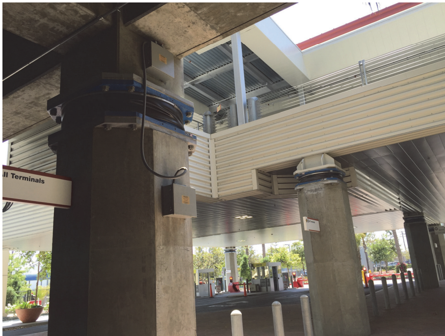
Figure 5-12 Seismic isolators on top of columns at an airport in Burbank, California.
