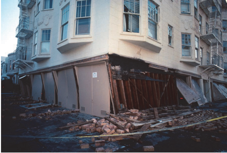
Figure 4-8 First story of an apartment building in San Francisco leaning to the side after the 1989 Loma Prieta Earthquake.
