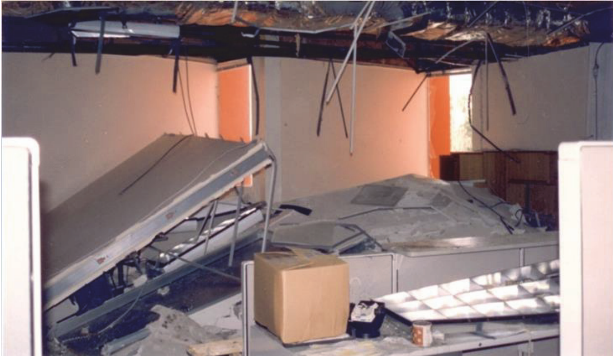
Figure 4-17 Failure of partitions, light fixtures, and ceilings in an office building damaged by the 1994 Northridge Earthquake (from FEMA E-74).
