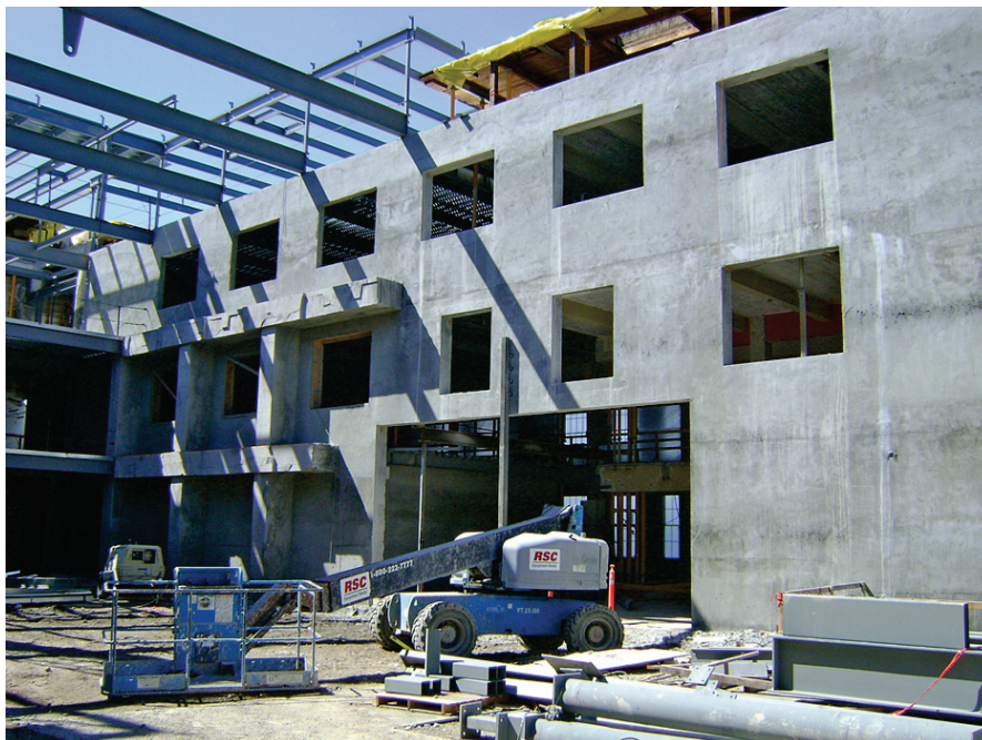
Figure 3-17 Illustration of the difficulty in identifying an isolated component boundary in a multistory reinforced concrete shear wall seismic-force-resisting system.
