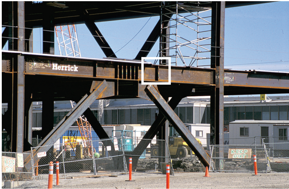
Figure 3-15 Illustration of proposed component boundary for the fuse element in a steel eccentrically braced frame seismic-force-resisting system (Engelhardt, 2007).
