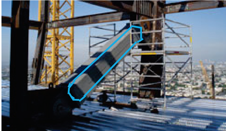
Figure E-4 Illustration of proposed component and definition of component boundary (Photo from Star Seismic).
