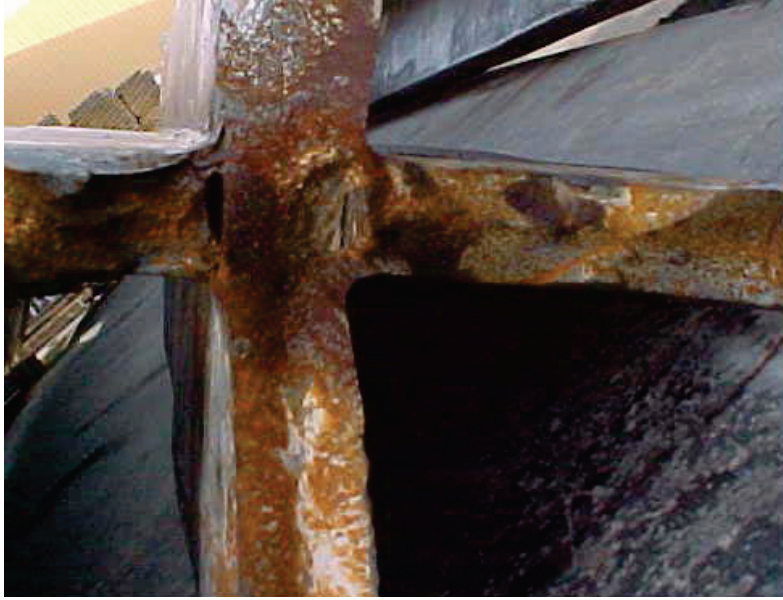
Figure E-10 Photo of steel core after fracture in buckling-restrained brace specimen (Merritt et al., 2003a).
