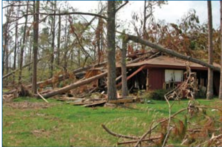
FIGURE 4-23: A home damaged by fallen trees during Hurricane Katrina (Diamondhead, MS) (SOURCE: FEMA 549)
