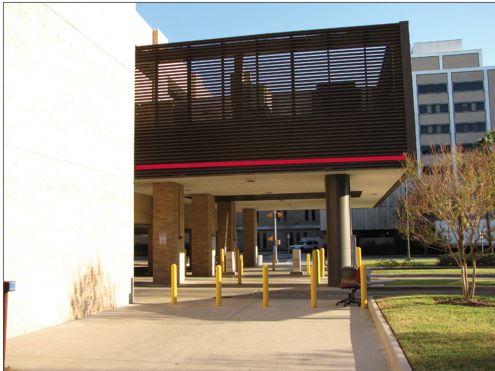
Figure 4-18. Emergency generator elevated above flood levels at the University of Texas Medical Branch, Hurricane Ike (Galveston, TX, 2008). The secondary switchgear shown in Figure 4-12 is located in the room to the left at approximately the same elevation as the emergency generator. The red line shows the location of the base of the generator.
