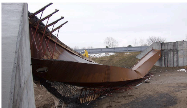
Fig. 25. Lateral-torsional buckling of Marcy Bridge [578].
